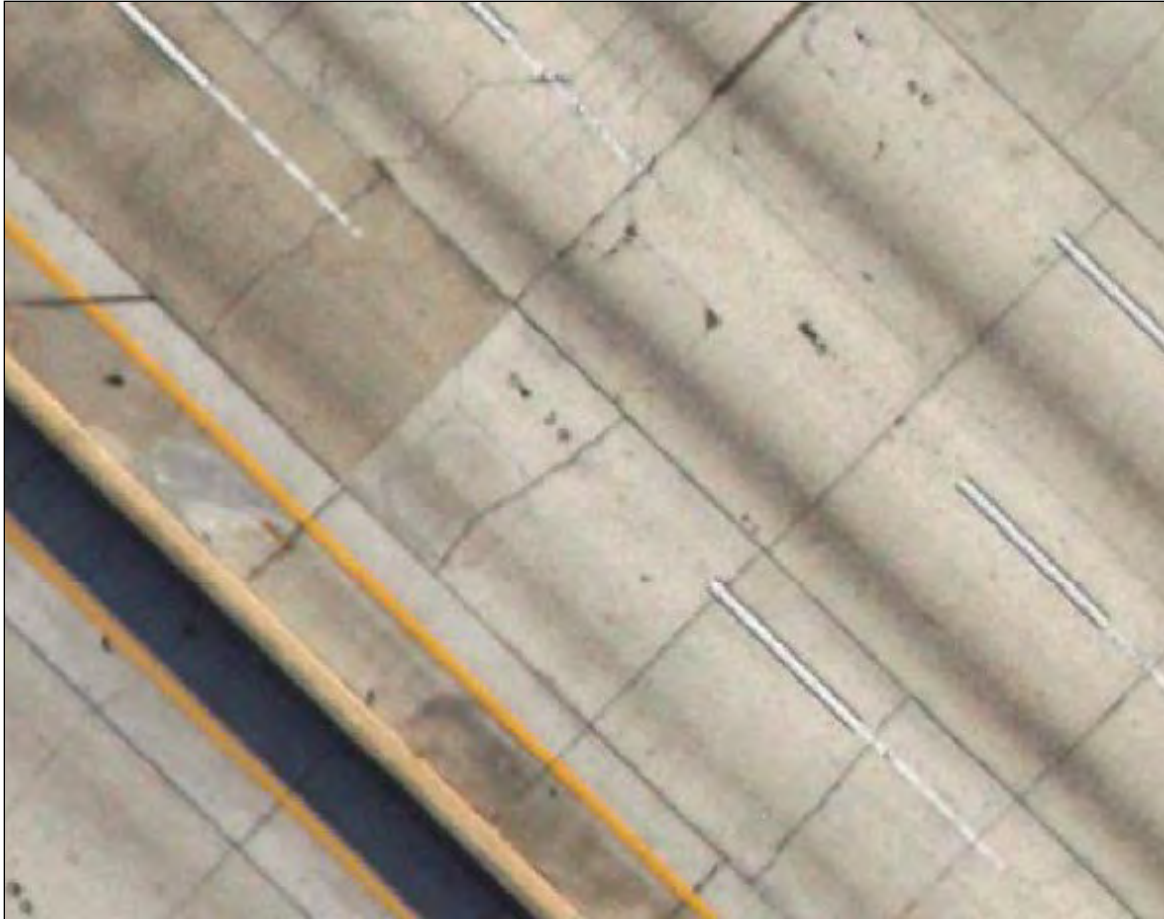
Figure 28. Image with vector file overlay used to quantify cracks, spalls, etc.
