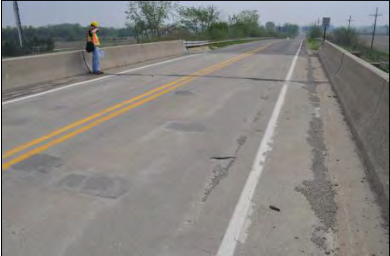
Figure 3-5: Willow Road bridge deck condition.
