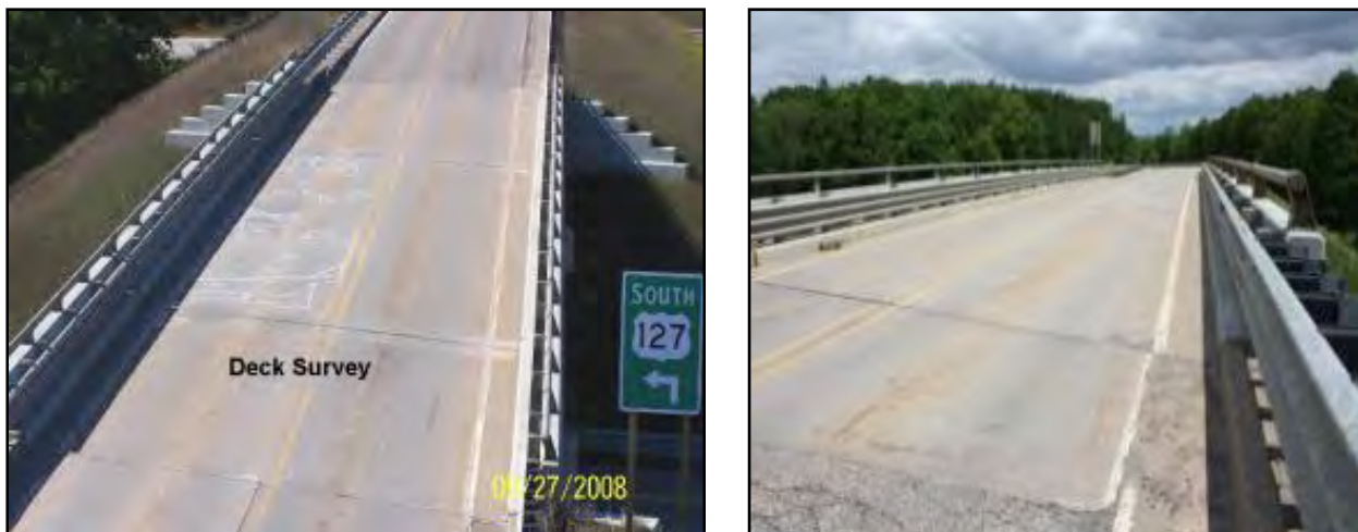
Figure 3-3: Mannsiding Road bridge NB deck condition in 2008 (a) and Mannsiding Road bridge NB deck condition in 2011 (b).
