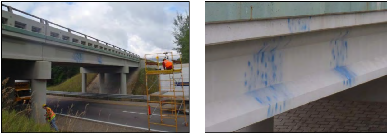
Figure 9-12: DIC setup at Mannsiding Road bridge and detail of girder with speckle patterns.
