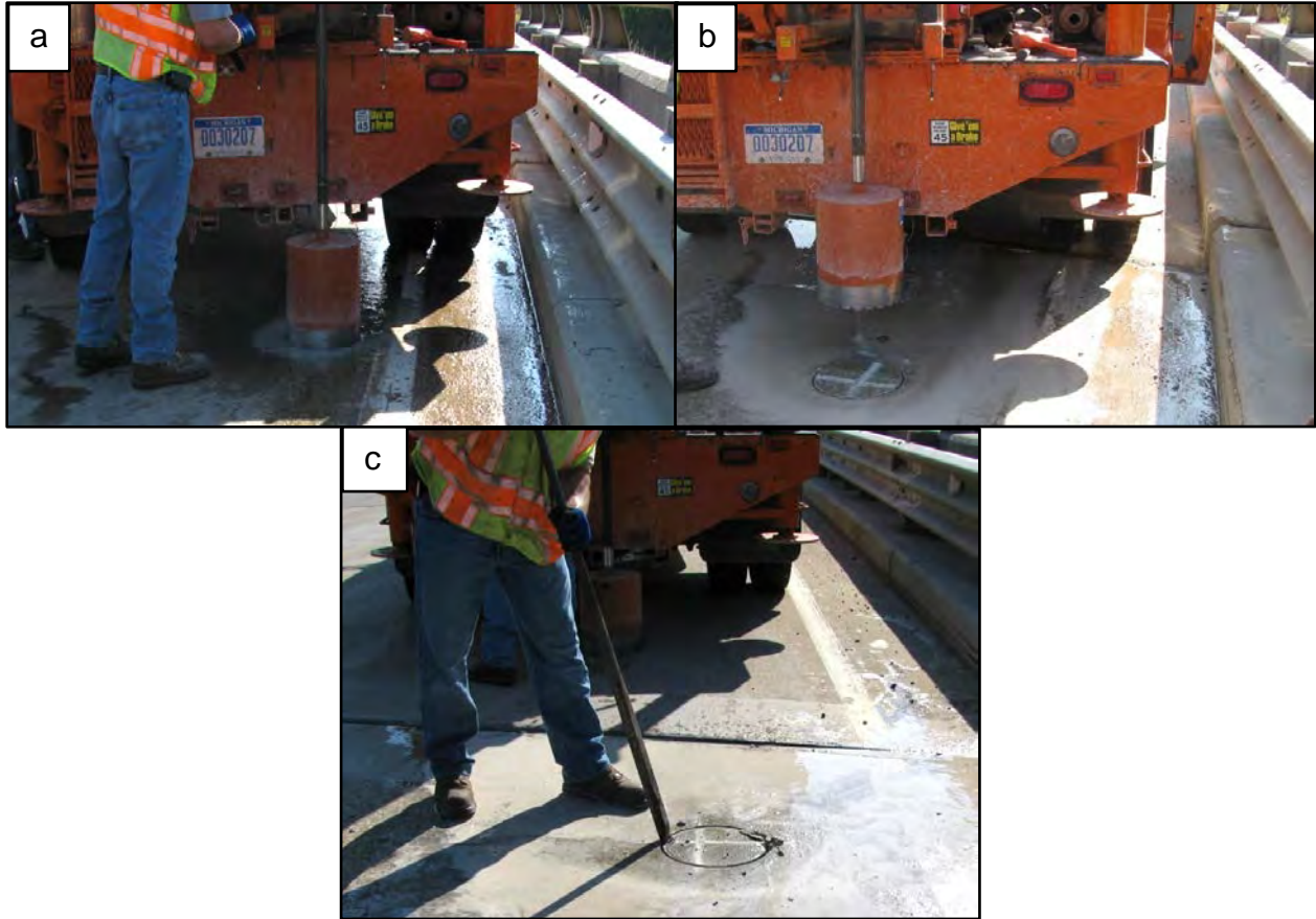
Figure 8-21: Drilling a core on the bridge deck (a), pulling out the drill (b), and pulling out the core with a pry bar (c).
