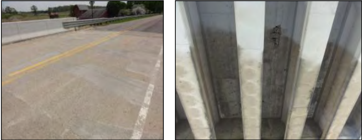
Figure 3-7: Freer Road bridge top and bottom surface conditions.
