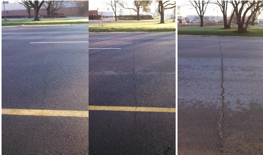
(a) Low (b) Medium (c) High Figure 6-1: Examples of low, medium, and high severity cracking
