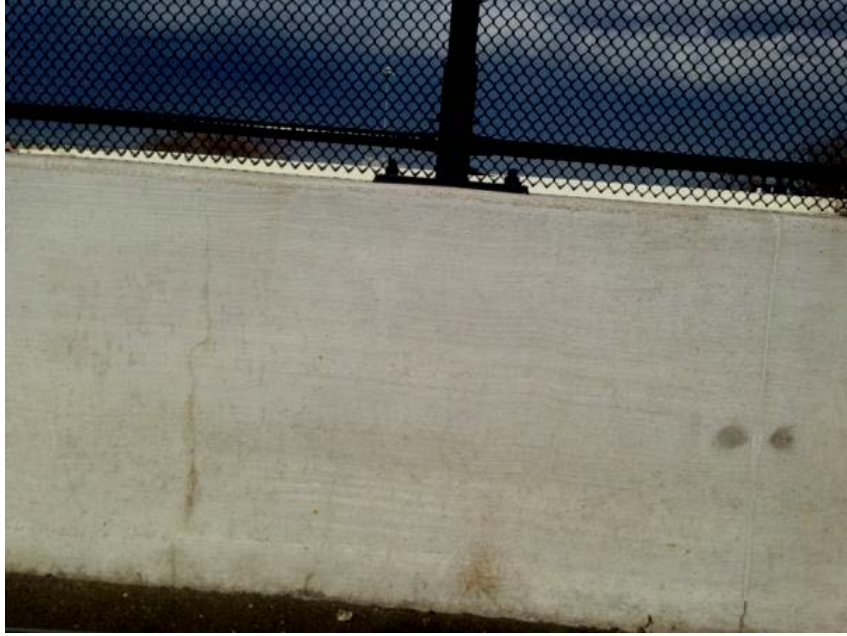
Figure 56: South Marginal north parapet mid-panel cracking (Photograph by Amy Kalabon)
