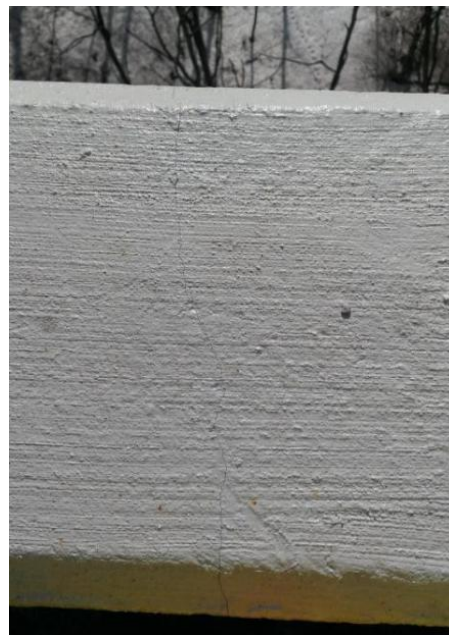
Figure 28: Crack along top of parapet (Photograph by Lauren Hedges)
