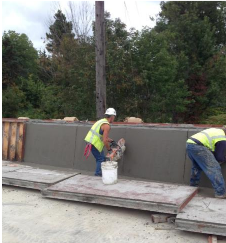
Figure 38: WB Paine Road north parapet performance of saw cuts (Photograph by Amy Kalabon)
