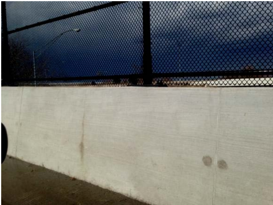
Figure 57: South Marginal north parapet mid-panel cracking (Photograph by Amy Kalabon)
