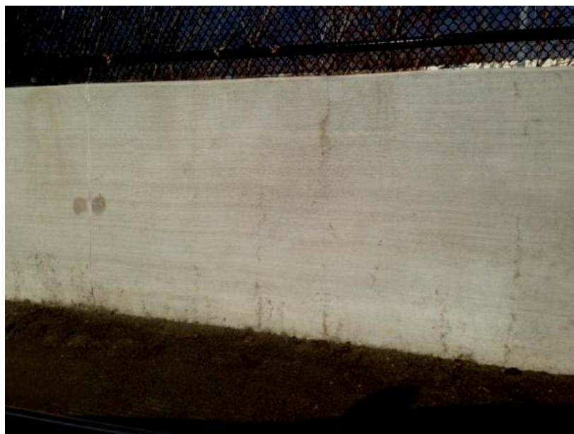
Figure 59: South Marginal north parapet small cracking (Photograph by Amy Kalabon)
