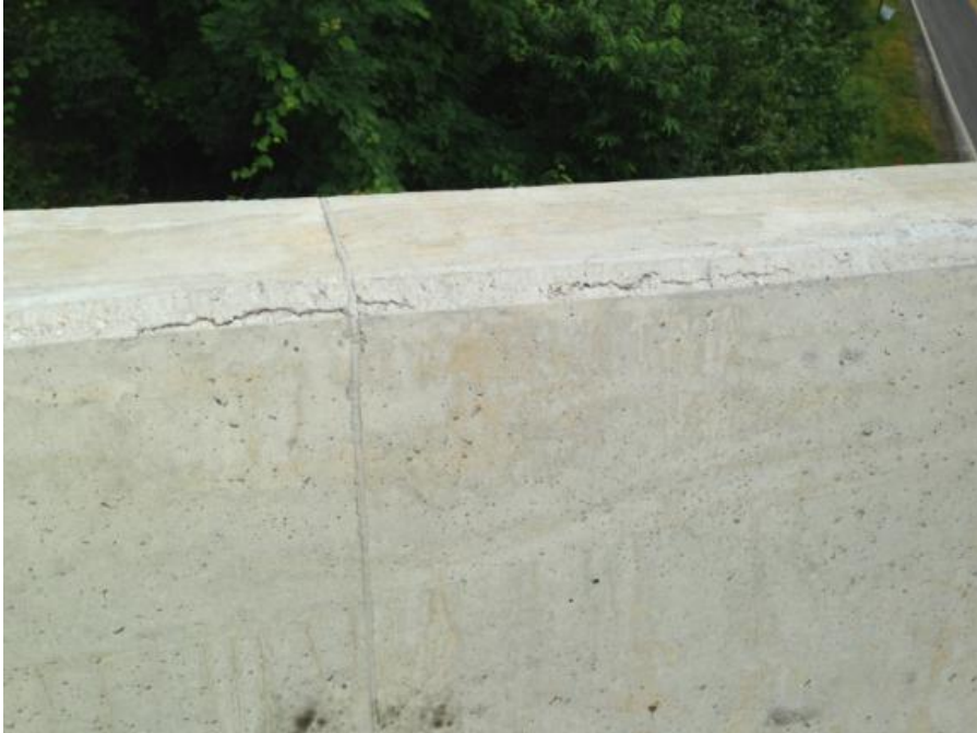
Figure 34: EB Hermitage Road north parapet surface cracks (Photograph by Amy Kalabon)
