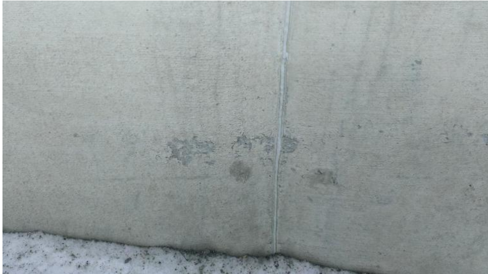
Figure 33: Spalling on EB Paine Road north parapet along location of horizontal reinforcement (Photograph by Lauren Hedges)
