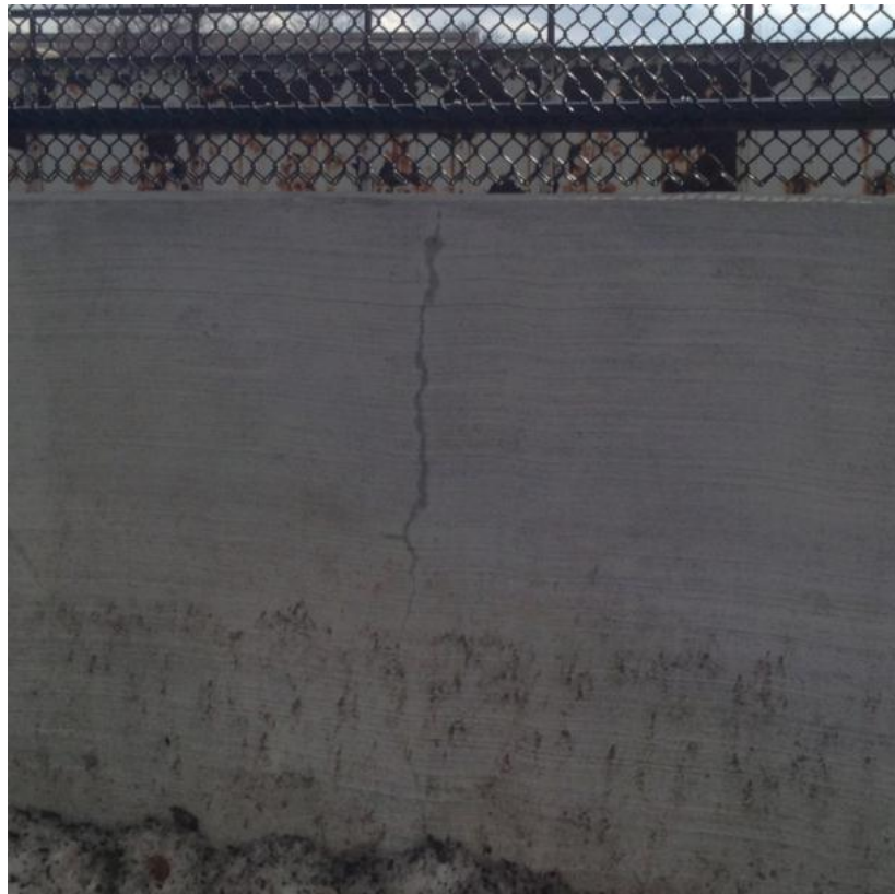
Figure 60: South Marginal south parapet mid-panel crack (Photograph by Amy Kalabon)
