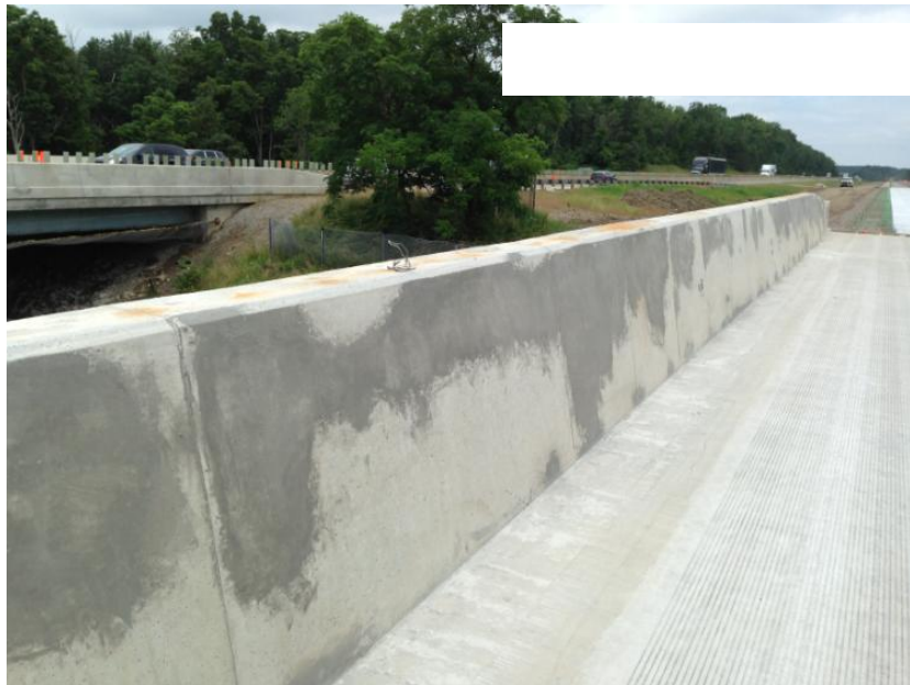
Figure 44: WB Paine Road rubbed south parapet (Photograph by Amy Kalabon)
