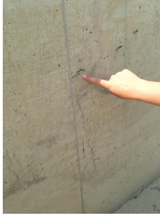
Figure 43: Surface cracks found on WB Paine Road south parapet (Photograph by Amy Kalabon)
