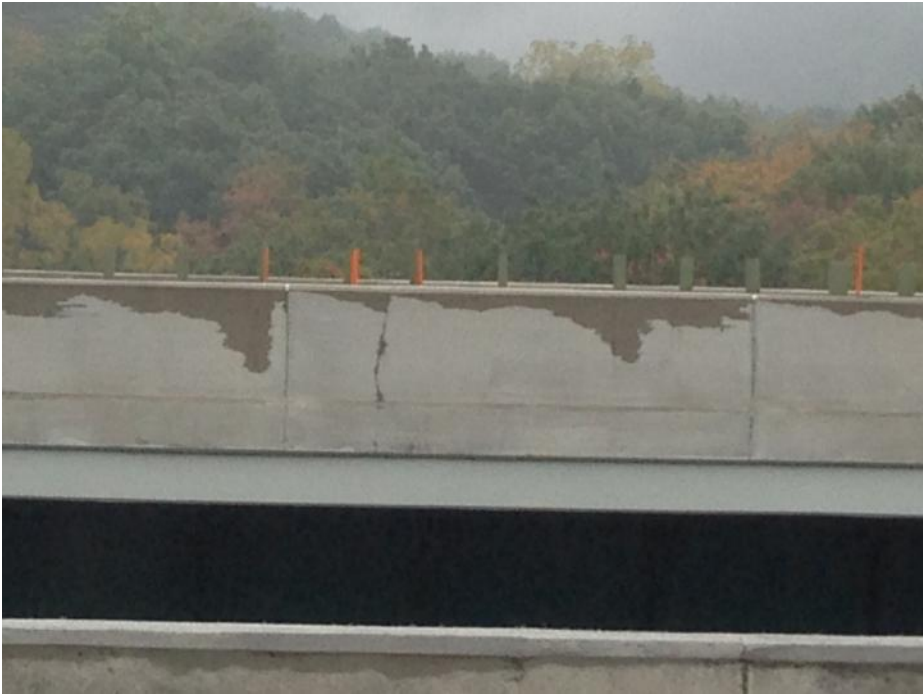
Figure 30: Looking at EB Paine Creek north parapet crack from adjacent bridge (Photograph by Lauren Hedges)
