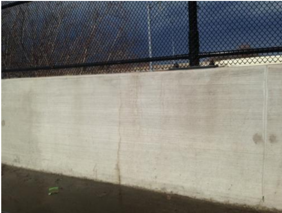
Figure 55: South Marginal north parapet mid-panel cracking (Photograph by Amy Kalabon)
