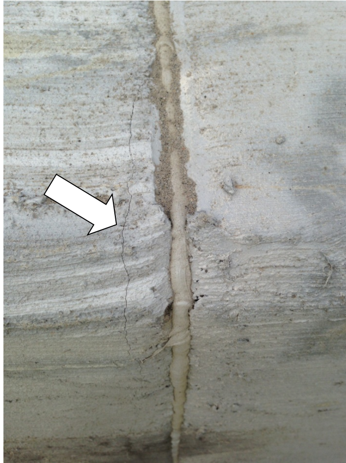
Figure 45: WB Paine Creek north parapet crack looking down from top of parapet (Photograph by Amy Kalabon)
