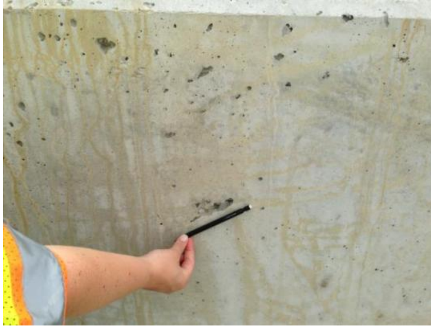
Figure 49: WB Paine Creek south parapet holes on the surface (Photograph by Amy Kalabon)
