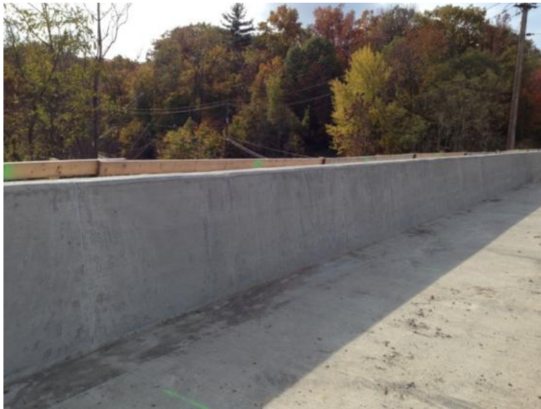
Figure 36: EB Hermitage south parapet condition (Photograph by Amy Kalabon)
