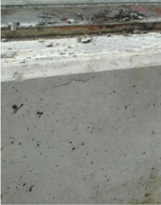
Figure 42: WB Paine Road south parapet bug holes (Photograph by Amy Kalabon)
