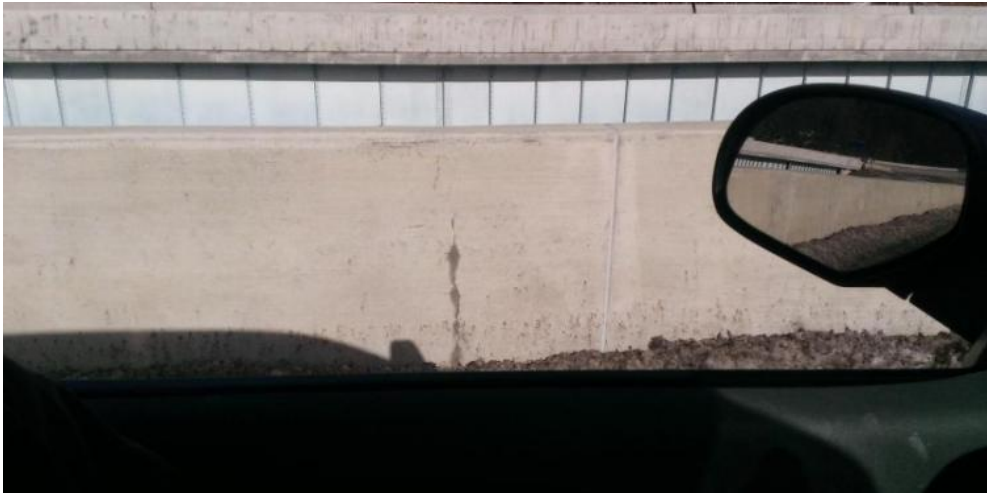
Figure 29: EB Paine Creek north parapet crack near control joint (Photograph by Lauren Hedges)
