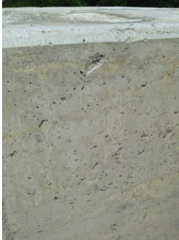
Figure 35: EB Hermitage Road north parapet typical bug holes (Photograph by Amy Kalabon)
