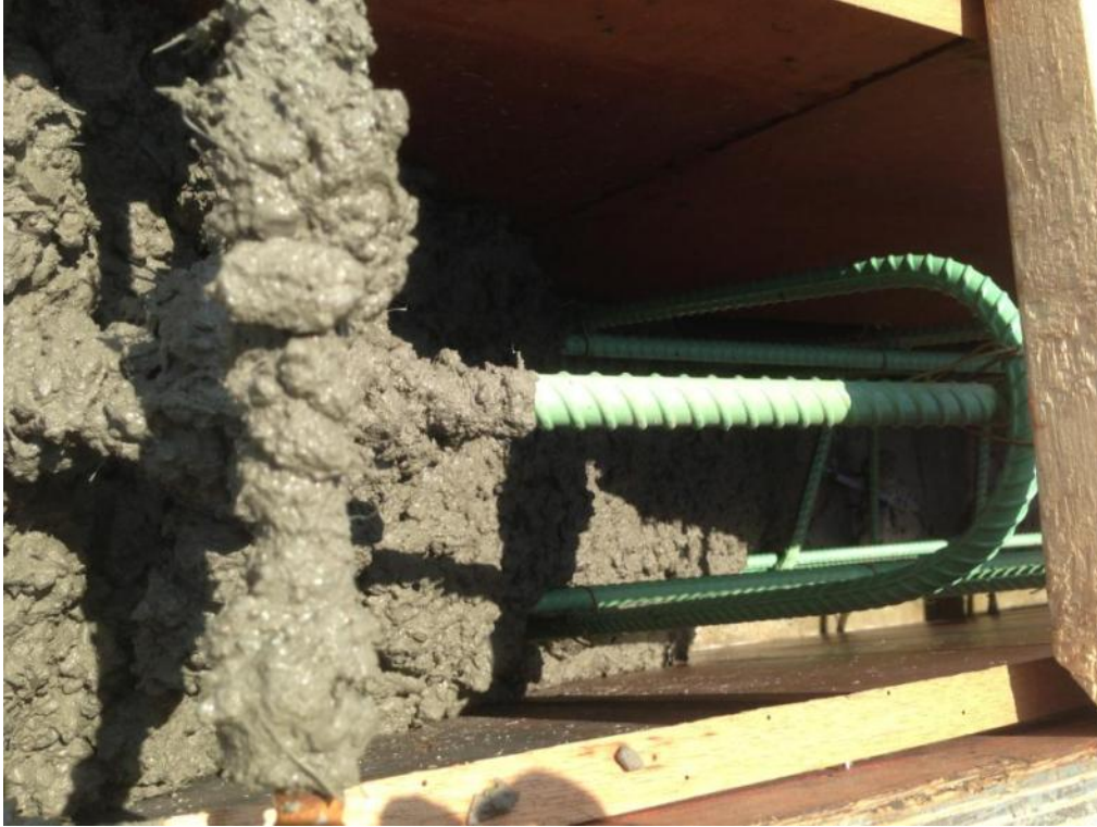
Figure 41: Consolidation of the concrete on WB Paine Road south parapet (Photograph by Amy Kalabon)
