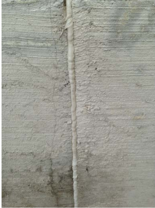
Figure 47: WB Paine Creek north parapet crack zoomed in view (Photograph by Amy Kalabon)
