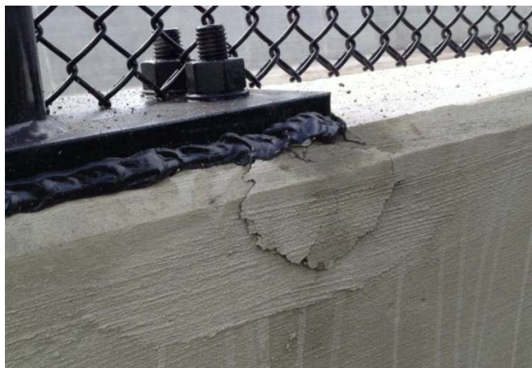
Figure 53: South Marginal north parapet crack at VPF post base plate (Photograph by Amy Kalabon)
