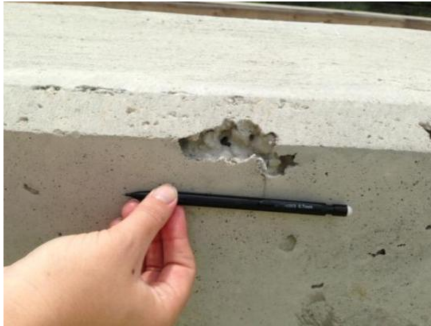
Figure 48: WB Paine Creek south parapet poor consolidation at the surface (Photograph by Amy Kalabon)
