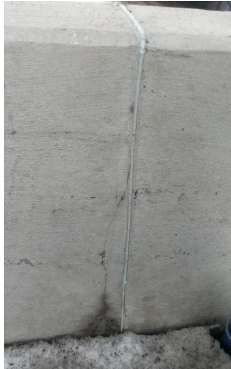
Figure 31: EB Paine Road north parapet crack propagating out of control joint (Photograph by Lauren Hedges)
