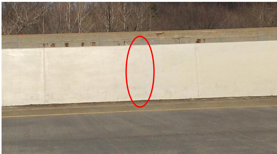
Figure 26: EB Big Creek Bridge North Parapet Crack (Photograph by Lauren Hedges)
