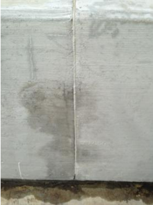
Figure 46: WB Paine Creek north parapet crack (Photograph by Amy Kalabon)
