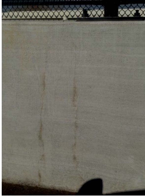
Figure 58: South Marginal north parapet mid-panel cracking (Photograph by Amy Kalabon)
