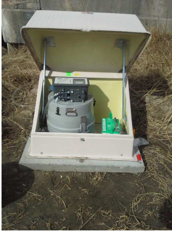
Figure 2.3 Autosampler installed at Highway 77 over Rock Creek site
