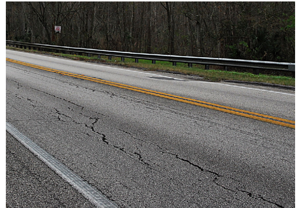
Cracking is an early step in the decay of a road surface. It leads to spalling and potholing, often requiring repeated repair.
