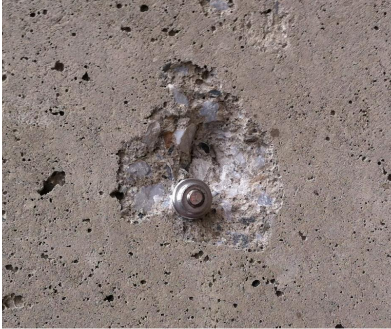
Figure 7 Powder Actuated Faster Caused Concrete to Burst (VTrans 2014)
