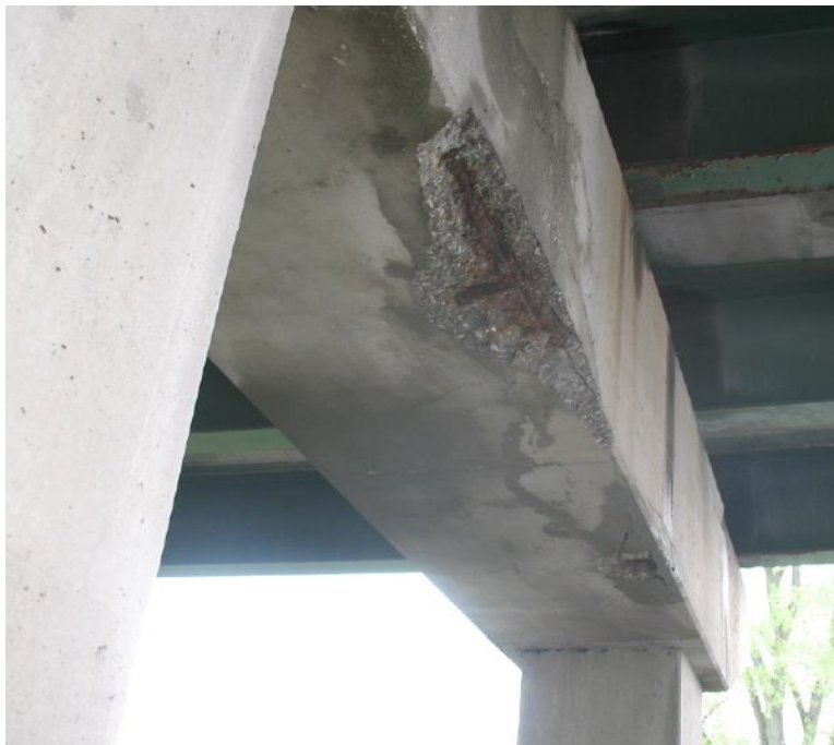
Figure 3 Concrete distress in pier bent (VTrans 2010)
