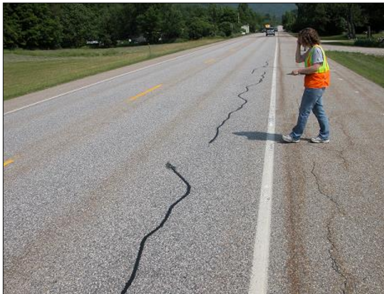
Figure 6 Fatigue cracking (Test Site 2, year 10)
