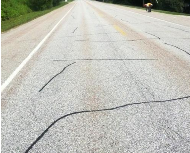
Figure 8 Example of transverse cracking (among others), within test site 1.
