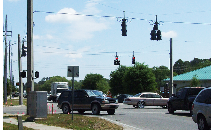
Above: The unobtrusive traffic control box at the left of this image integrates timing schedules, crossing request buttons, and in-road sensors to improve the efficiency and safety of intersections.
