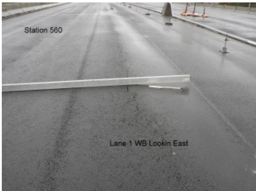
Figure 1. Picture showing heave present in the west bound lane of Route 2 at station 560.
