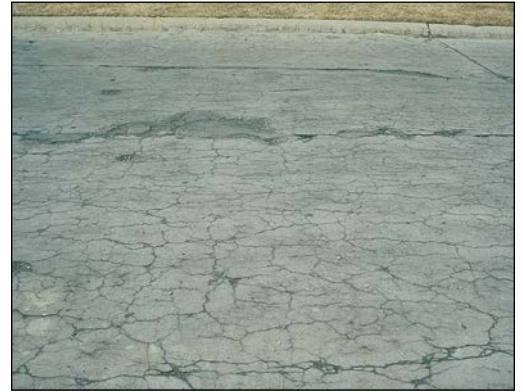
FIGURE 69 Distress Type JCP 8a—Map Cracking.
