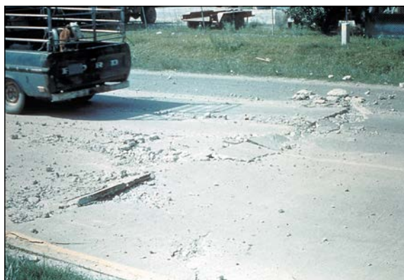
FIGURE 76 Distress Type JCP 11—A Blowup.
