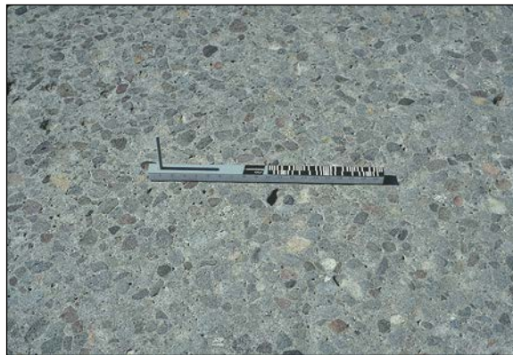
FIGURE 74 Distress Type JCP 10—A Popout.
