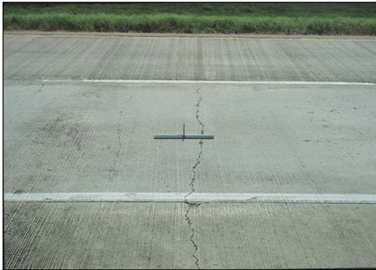
FIGURE 99 Distress Type CRCP 3—Moderate Severity Transverse Cracking.
