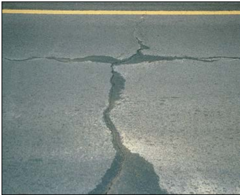
FIGURE 45 Distress Type ACP 15—Water Bleeding and Pumping.
