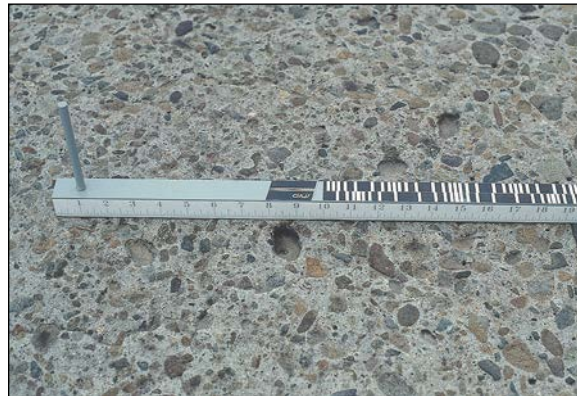
FIGURE 105 Distress Type CRCP 6—Popouts.
