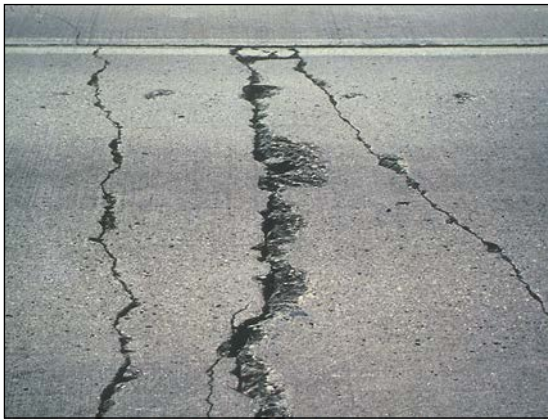
FIGURE 100 Distress Type CRCP 3—High Severity Transverse Cracking.
