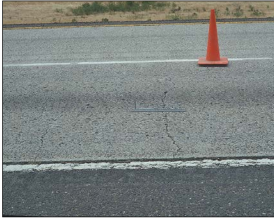
FIGURE 98 Distress Type CRCP 3—Low Severity Transverse Cracking.
