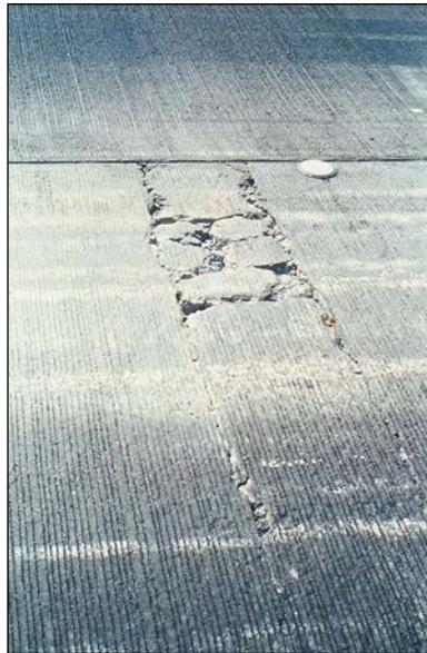
FIGURE 126 Distress Type CRCP 12—High Severity Punchouts.
