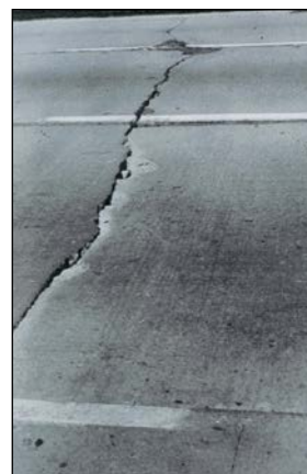
FIGURE 78 Distress Type JCP 12— Faulting of Transverse Cracks.
