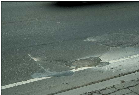
FIGURE 25 Distress Type ACP 7—High Severity Patch.
