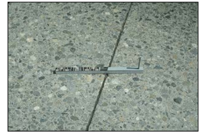
FIGURE 61 Distress Type JCP 5—Low Severity Joint Seal Damage.
