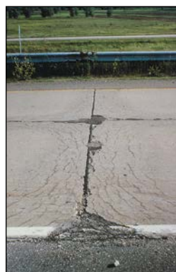
FIGURE 53 Distress Type JCP 2—High Severity “D” Cracking with Loose and Missing Material.
