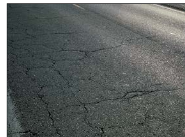
FIGURE 10 Distress Type ACP 2—High Severity Block Cracking.
