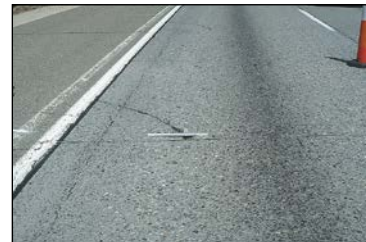
FIGURE 50 Distress Type JCP 1—Moderate Severity Corner Break.
