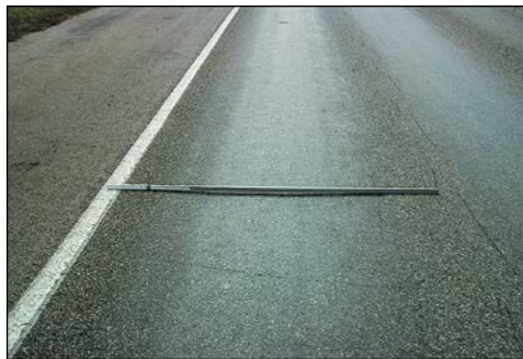
FIGURE 32 Distress Type ACP 9—Rutting.
