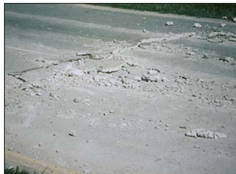
FIGURE 107 Distress Type CRCP 7—A Blowup.
