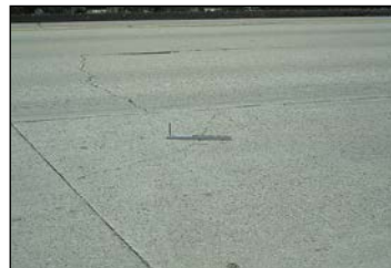
FIGURE 49 Distress Type JCP 1—Low Severity Corner Break.
