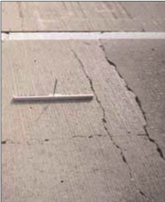
FIGURE 125 Distress Type CRCP 12—Moderate Severity Punchouts.
