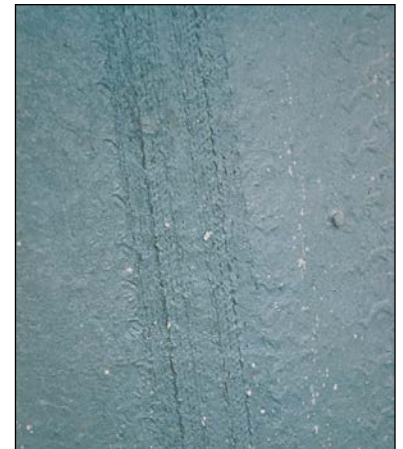
FIGURE 38 Distress Type ACP 11—Aggregate Obscured.
