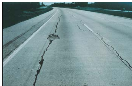
FIGURE 95 Distress Type CRCP 2—High Severity Longitudinal Cracking.
