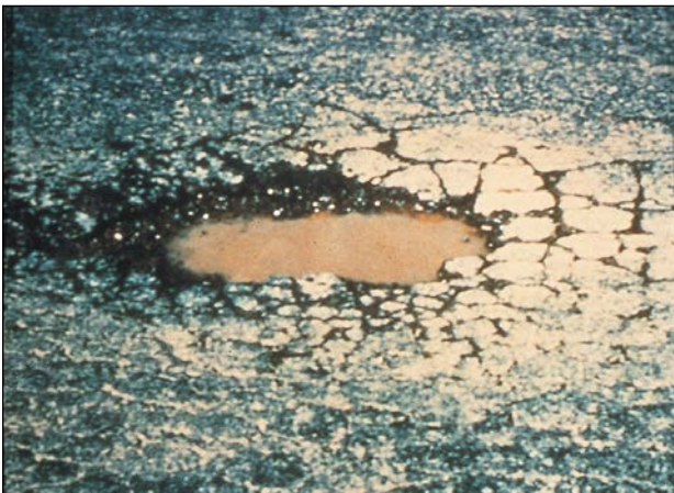
FIGURE 30 Distress Type ACP 8—High Severity Pothole, Close-up View.
