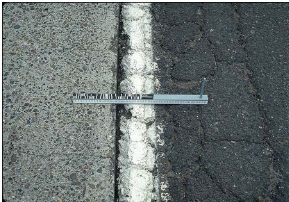
FIGURE 117 Distress Type CRCP 10—Close-up View of a Lane-to-Shoulder Separation.
