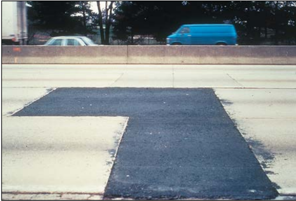
FIGURE 86 Distress Type JCP 15—Large, Low Severity AC Patch.
