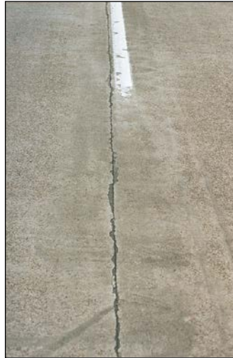
FIGURE 129 Distress Type CRCP 13— Low Severity Spalling of a Longitudinal Joint.
