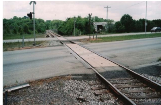
May, 2008, Slight Reveling of Asphalt Approaches
