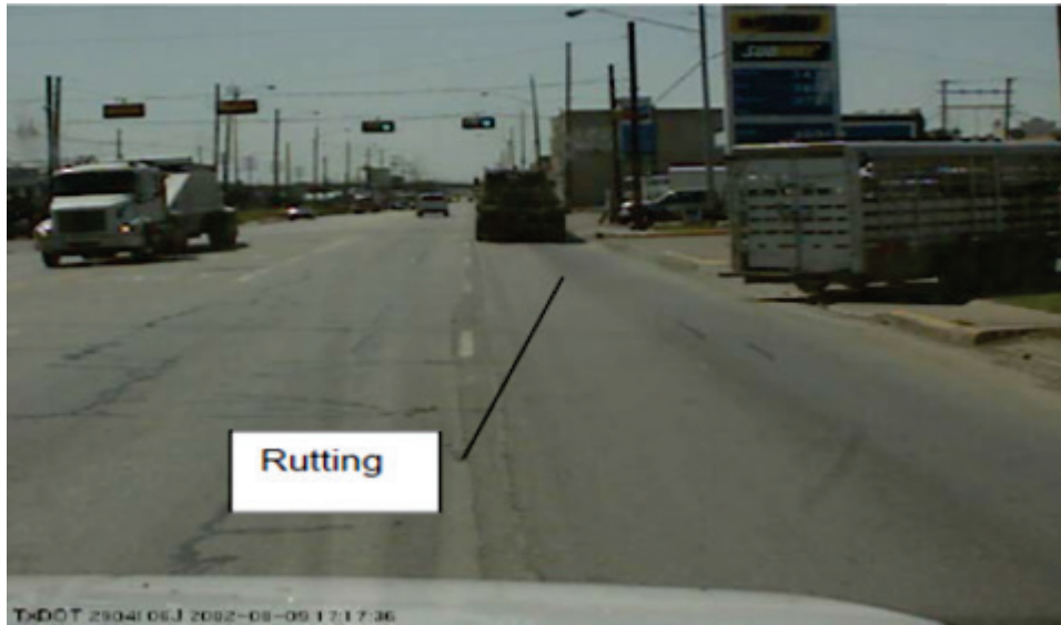
Figure 1-3. Surface Rutting on Anderson Street in Bryan District (over 0.5 inch Surface Rutting).
