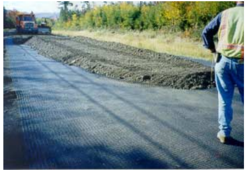
Pushing or Waving of Geogrid Material
