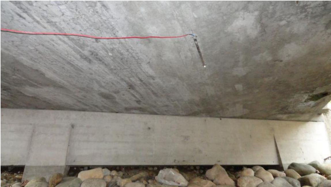
Figure 5 - One of two gages with extension on approach slab.
