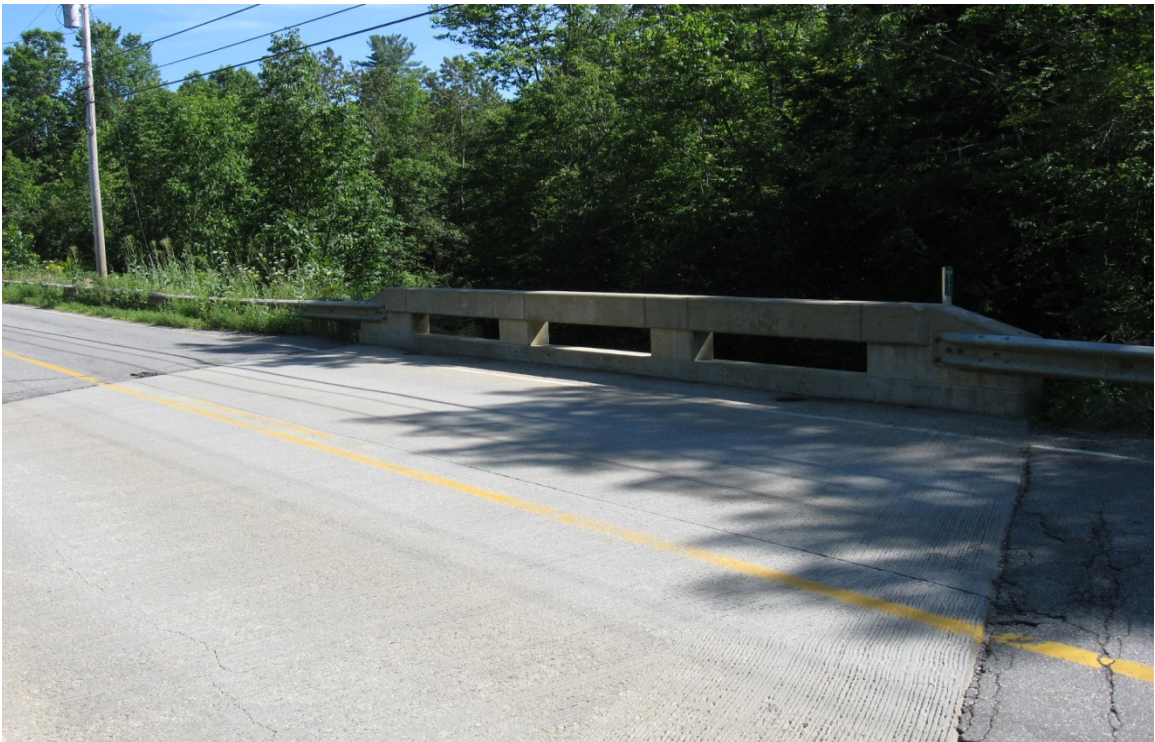
Figure 32 - Photo of Carmel Bridge #5191 Rail from Bridge Visit Conducted in July 2010
