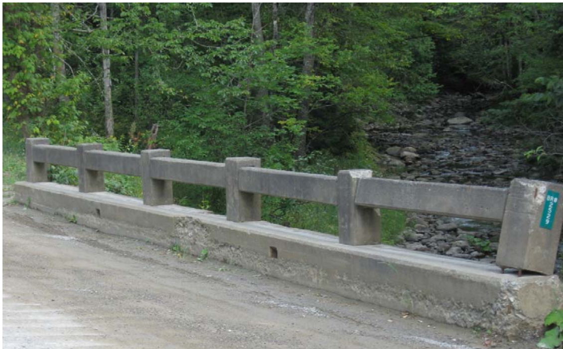
Figure 28 – Photo of the Rail on Albion Bridge #2529 from Bridge Visit in August 2010
