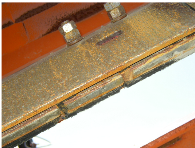
Photo 3: 2007 Photo of Failed Cutting Edge
