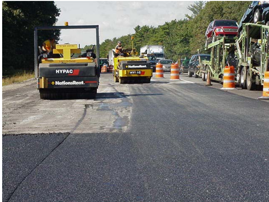
Photo 6: Route 1 and Turnpike Spur, right lane of T-section
