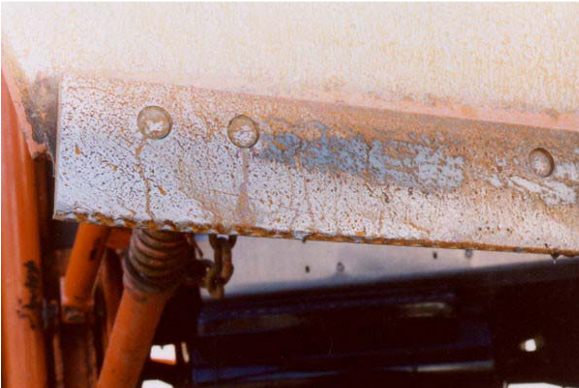
Figure 4. View of Remaining Carbide Inserts after Plowing Several Storms
