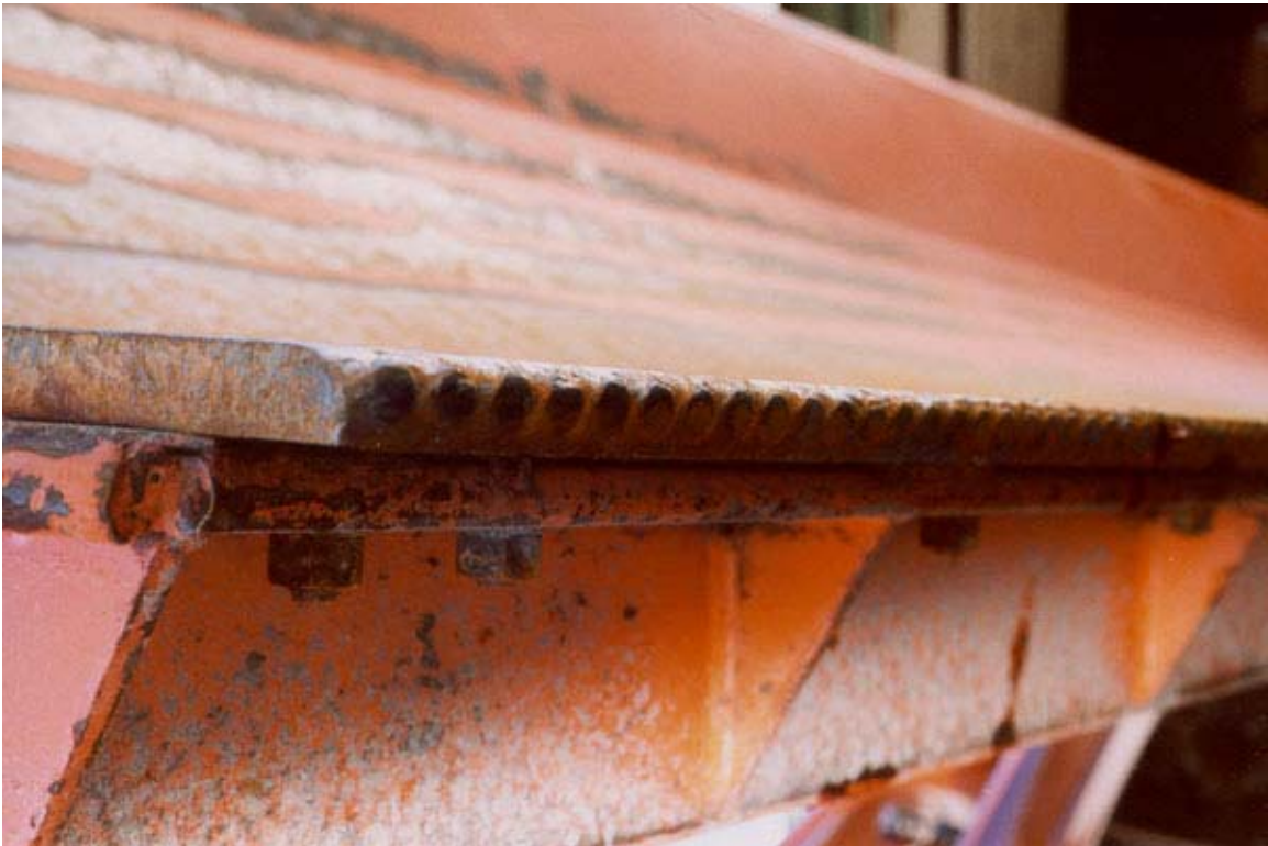
Figure 3. Test Blades as seen from the Road Perspective
