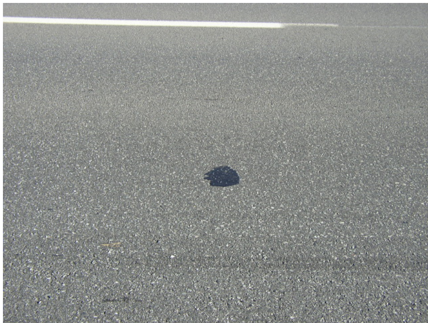
Photo 6. Surface defect on Bridge # 1558
