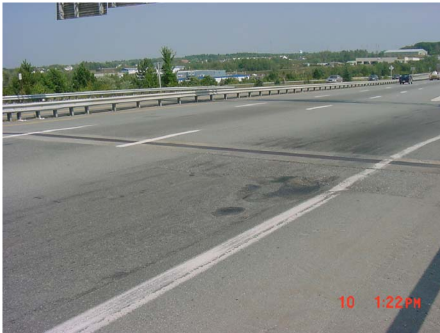
Photo 4. Bridge # 1558 patch area on exit ramp
