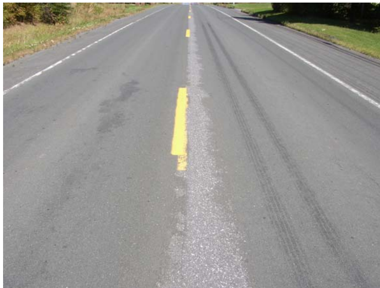
Photo 8: Section 5 Micro-Surface Pavement Condition; September, 2005.
