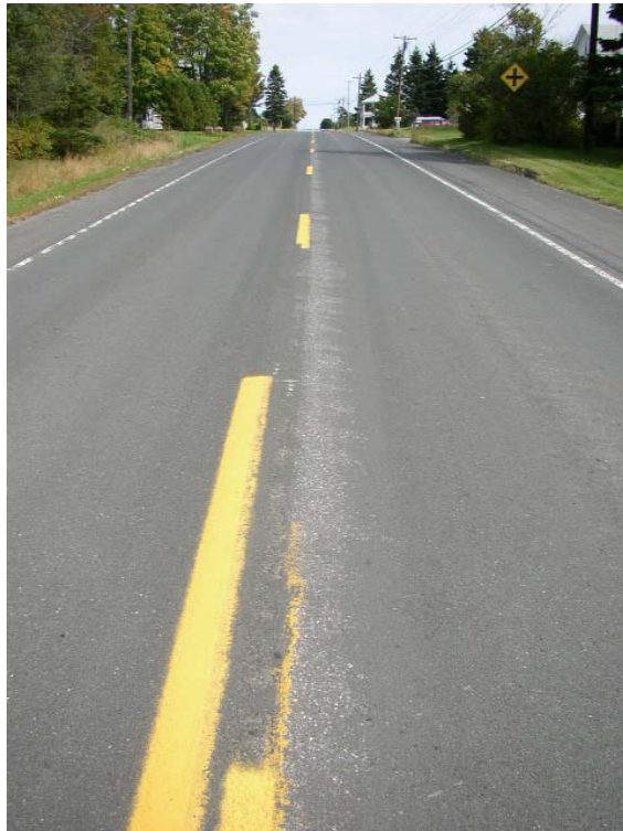
Photo 7: Section 5 Micro-Surface Pavement Condition; September, 2003.
