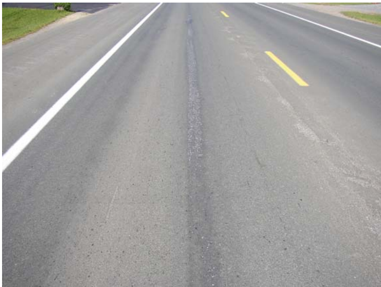
Photo 3: Section 1 Micro-Surface Centerline and Quarter Point Plow Abrasion; September, 2005.
