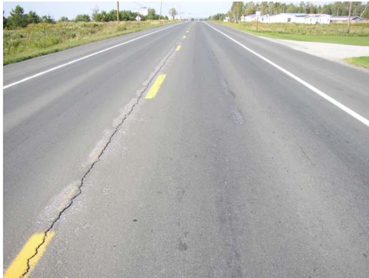
Photo 4: Section 4 Micro-Surface Centerline and Quarter Point Plow Abrasion; September, 2005.
