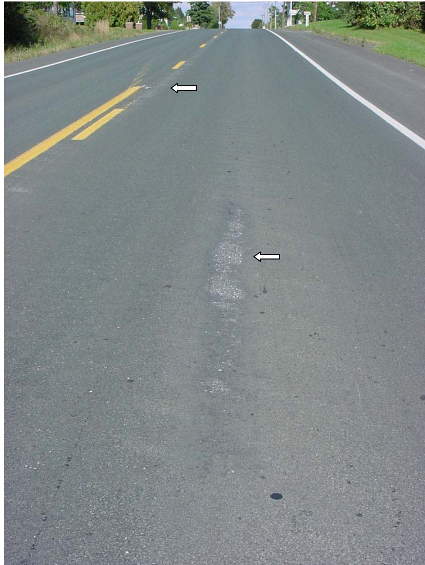
Figure 2: Between Wheel-Path and Centerline Plow Wear, Limestone Project.
