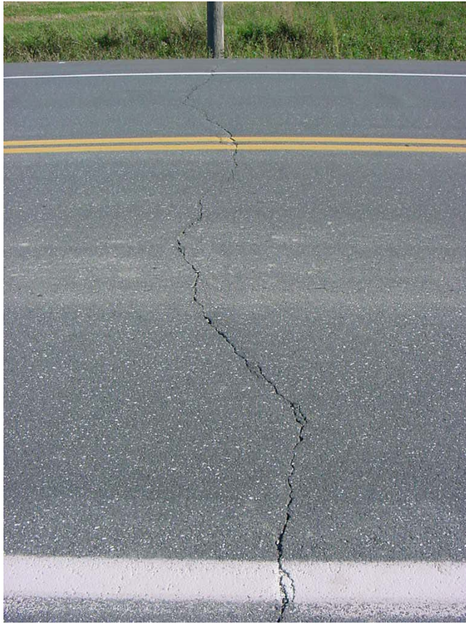
Figure 19: Control Section 6 transverse crack
