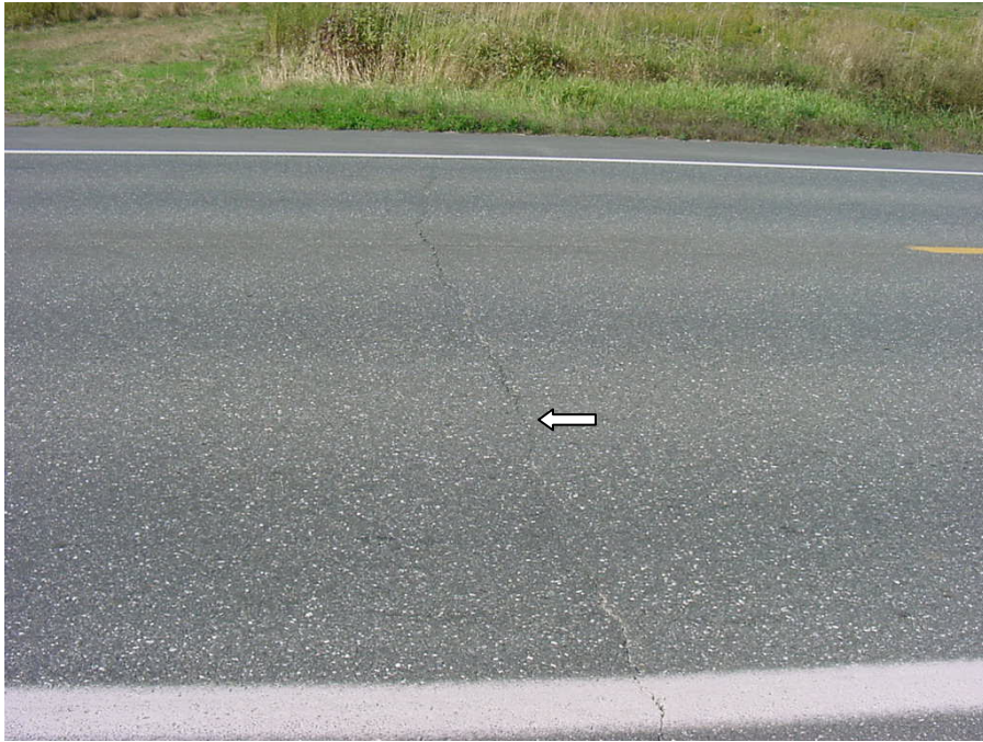
Figure 17: Control Section 3 transverse crack.
