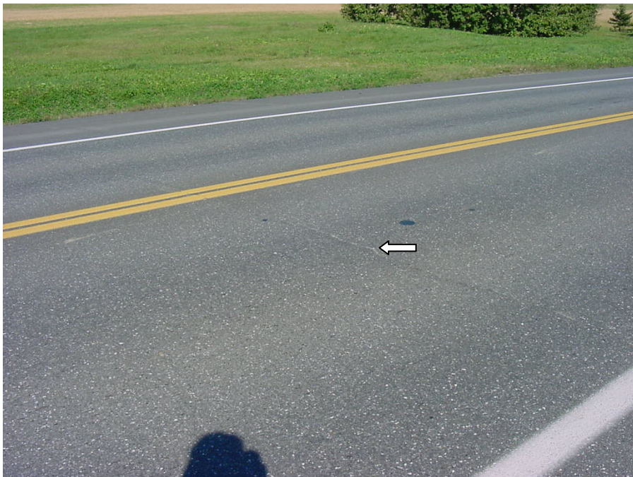
Figure 16: Control Section 2 transverse crack
