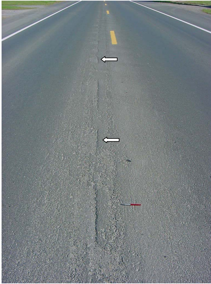
Figure 15: Micro-Surface Section 1 snow plow wear
