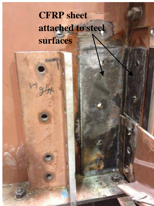
Figure 3.15: Trial 2: view of the interior face of the girder's web before application of the angles-with-plate-with-CFRP retrofit measure
