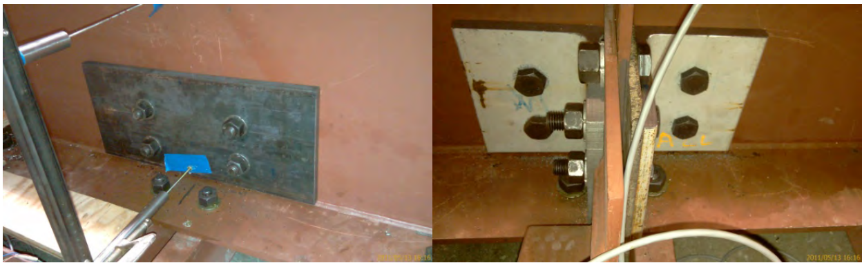
Figure 3.3: Angles-with-plate repair installed in the bottom web gap of the 2.8 m (9.3 ft) girder model
