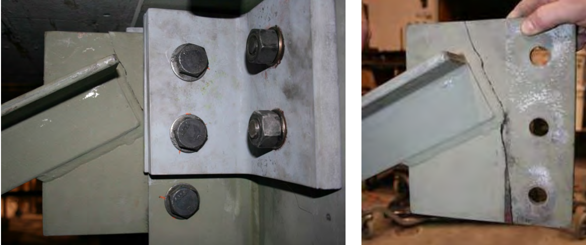
Figure 4.6: North cross frame failure during Trial 4N
