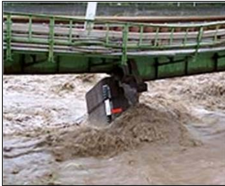
Figure 2. A bridge pier collapsing due to scour during flood flows caused by a typhoon (Akabane River, Japan, September 2004).
