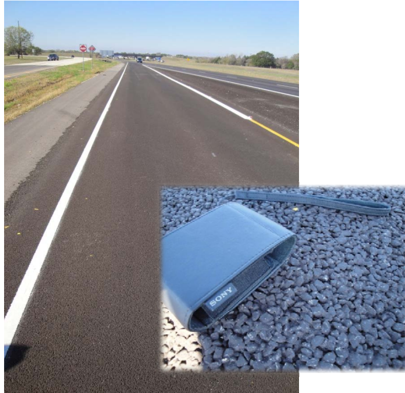
Figure 22. Project and Surface Texture (Bryan-Fine PFC).
