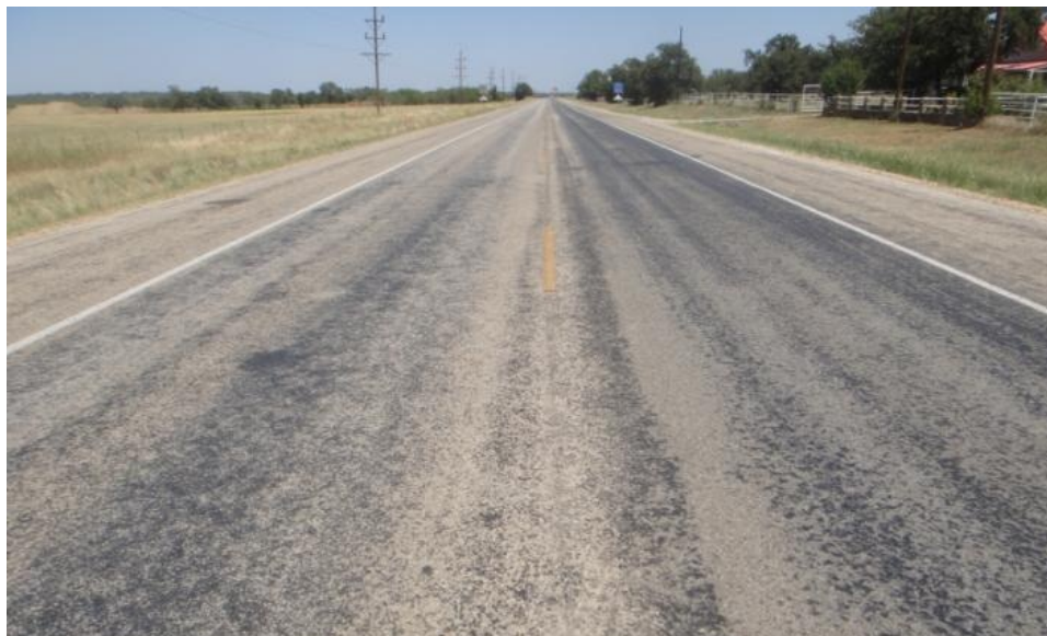
Figure 24. Flushing Surface Treatment (Brownwood-Fine PFC).
