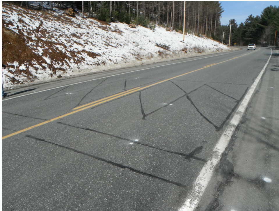
Figure 2 An example of a Manufactured Cracked Test Site
