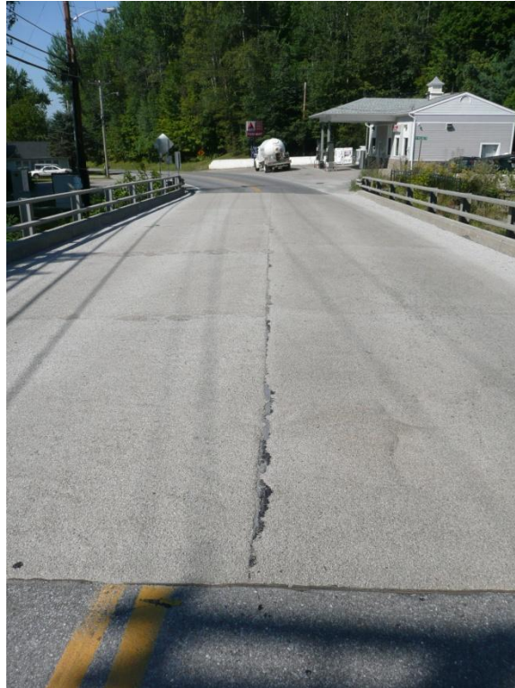
Figure 17 Application after installation in 2008
