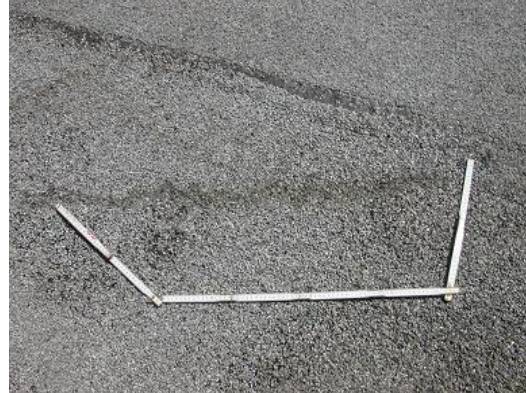
Figure 13: Water seeping through 1 st lift of overlay
