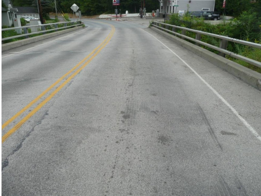
Figure 18 The darken wheel paths show where the aggregate has been stripped, exposing the underlying epoxy (2010).
