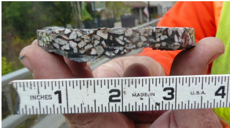
Figure 19 Core of the overlay.
