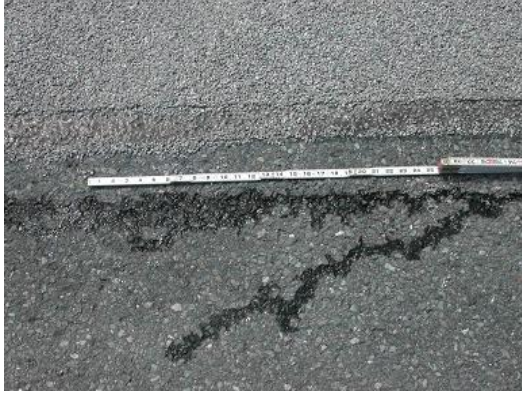
Figure 12: Water leaking from the centerline joint
