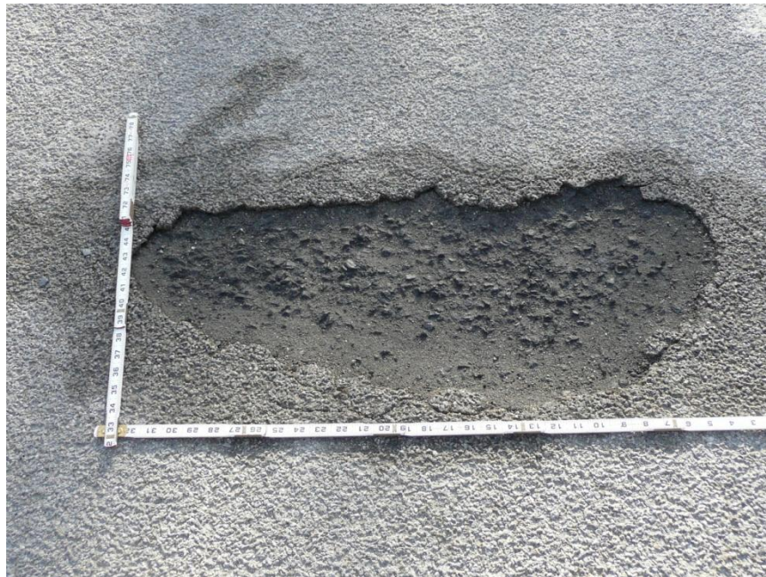
Figure 14 An example of a pothole. The underlying pavement was lifted out with the overlay.
