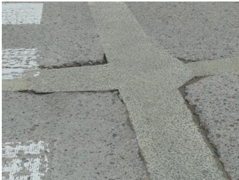
Figure 15 Condition of some repair areas following the second winter of service life (2011).
