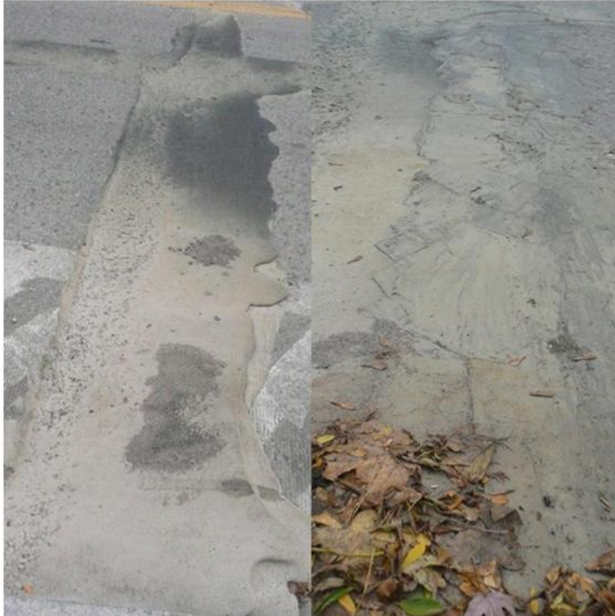
Figure 8 Side by side comparison of an overfilled joint (left) and the same joint after removal of material (right)
