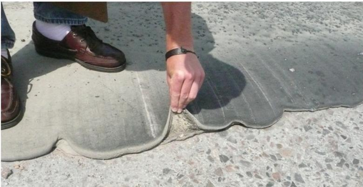
Figure 7 Excessive placement of TechCrete on an inclined joint
