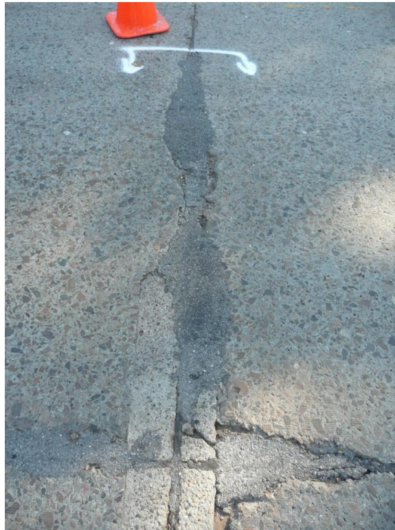
Figure 4 Typical concrete joint deterioration prior to repair
