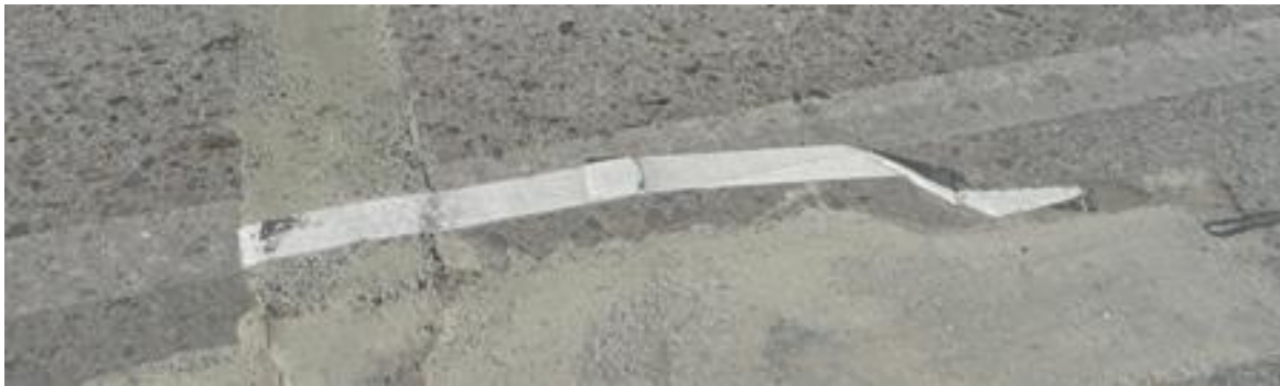
Figure 13: Tape markings adhered to TechCrete but not to the concrete
