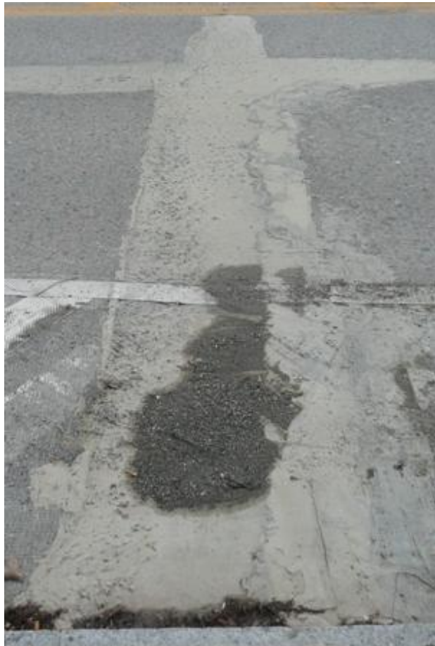
Figure 12: Condition of joint following first winter season
