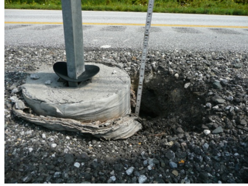
Figure 10: Erosion around the post foundation
