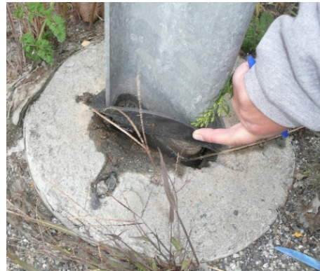
Figure 8: Debris and water build-up in and around the posts
