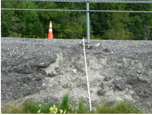
Figure 9: Erosion of the bank - median side
