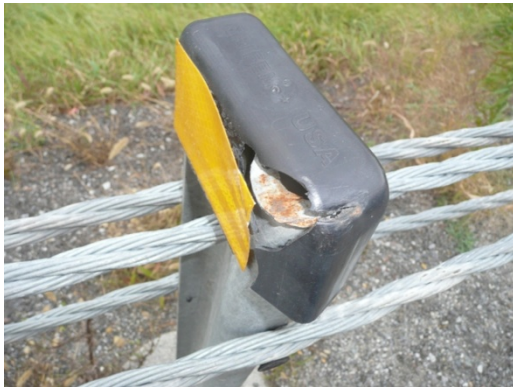
Figure 7: Cracked post cap
