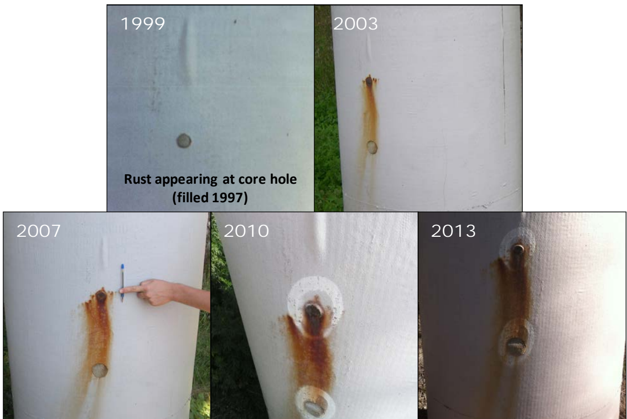
Figure 8 Core hole (filled in 1997) in Column #1 under pier #1, over time.
