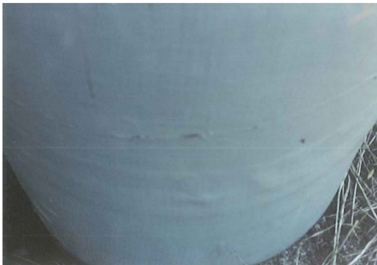
Figure 6 Slight Separation, not substantial in length or depth (1999).
