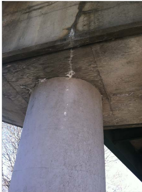
Figure 9 Chlorides leaching onto column.
