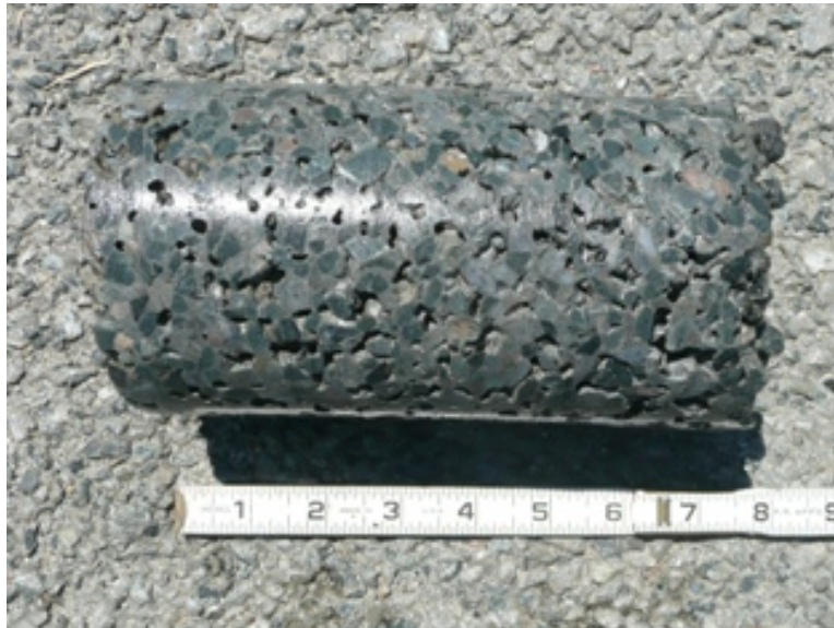
Figure 10. Core 6, taken from a visually and audibly sound but clogged location at the exit.
