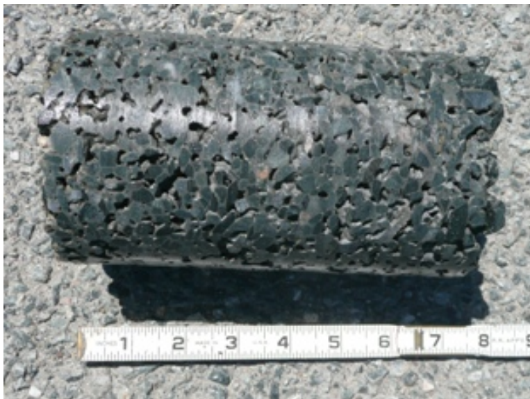
Figure 9. Core 5, taken from a visually and audibly sound but clogged location at the entrance.
