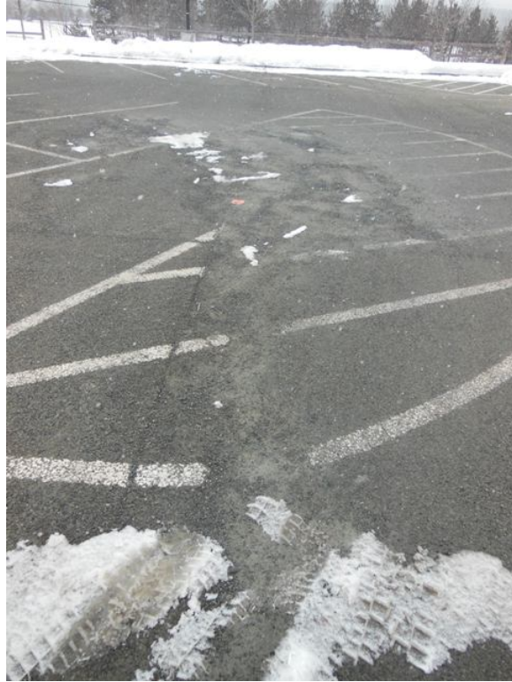
Figure 12. Deterioration in the gore area of the front portion of the lot after five winter seasons.
