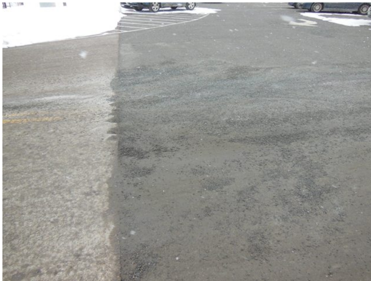
Figure 13. Deterioration at the transition between the bituminous drive (left) and porous concrete lot (right) after five winter seasons.
