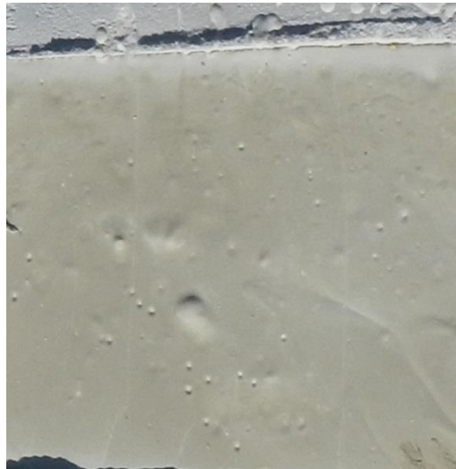
Figure 0.1 CSA cement with surface cracks
