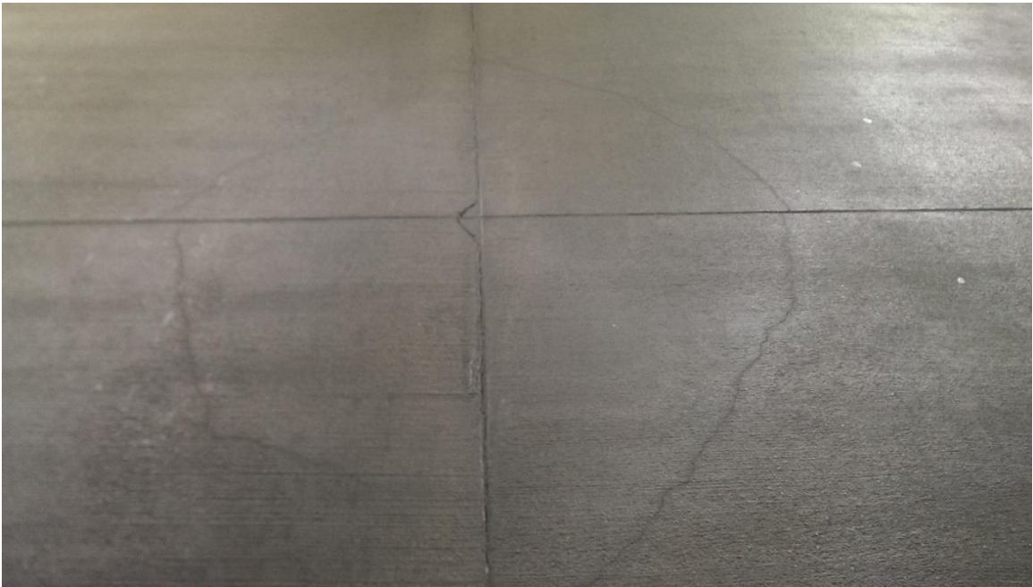
Figure 2.2 Pavement with surface cracks
