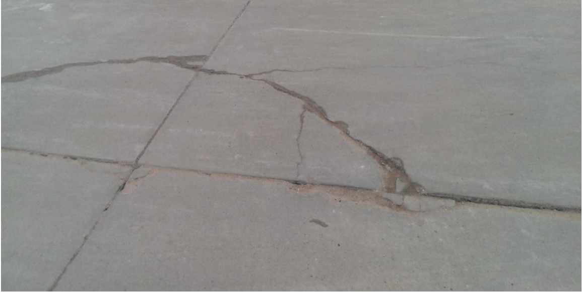
Figure 2.1 Pavement with surface cracks
