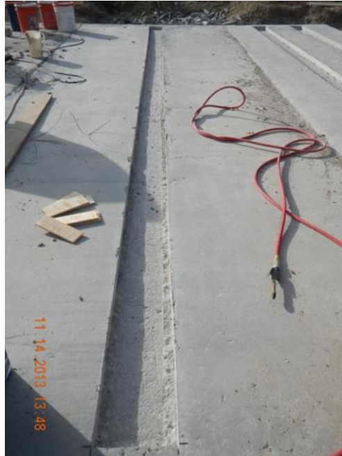
Figure 0.12 Concrete void strips before repair application
