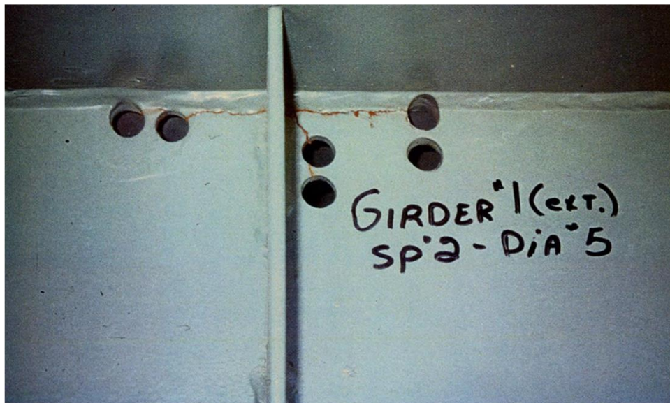
Figure 1.2 Retrofitted fatigue crack of highway steel-girder bridge with re-initiation. Figure from FHWA Publication No. FHWA-IF-13-020
