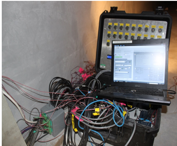
Figure 3-20 Data Collection Unit in Interior of HCB
