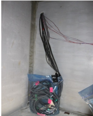
Figure 3-19 Entry of Data Cables into Interior of HCB
