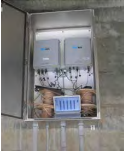
b) Dataloggers at Abutment
