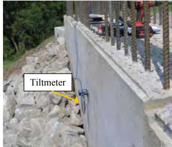
Figure 3-50: Tiltmeter Location Abutment at East Montpelier Bridge
