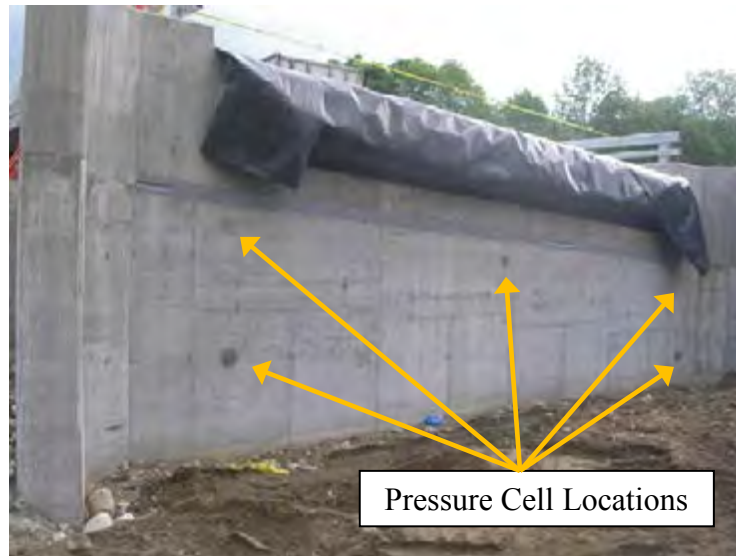
Figure 3-44: Abutment Pressure Cell during Backfilling at Stockbridge Bridge (Top Two Rows of Cells)
