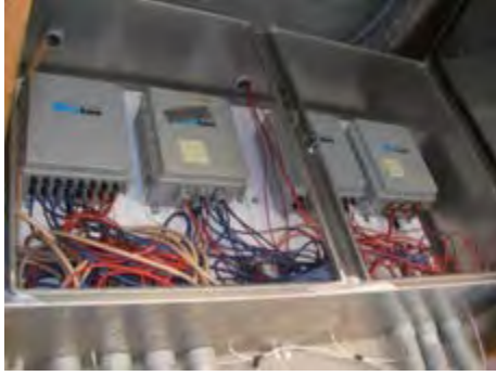
a) Multiplexers at Abutment
