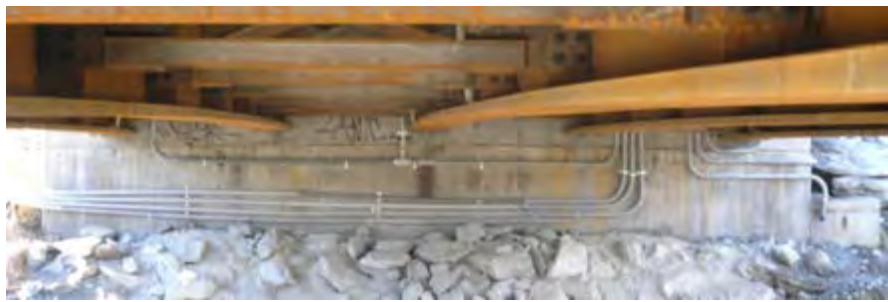
Figure 3-2: Cable Routing on the Abutment
