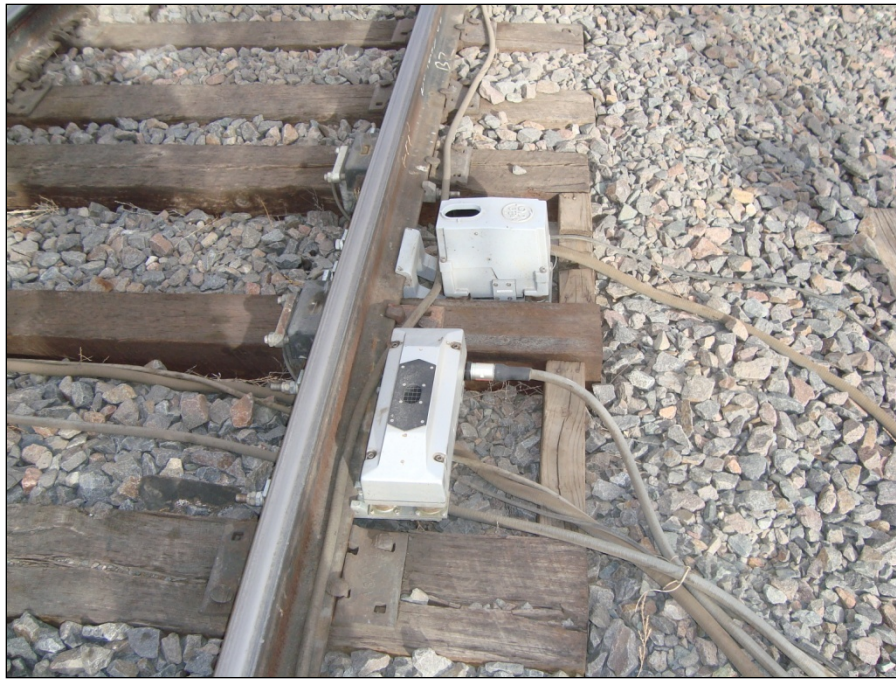
Figure 4. Wheel Temperature Detector Installation at FAST
