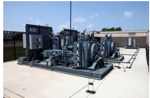
Figure 2(d). CNG Compressor
