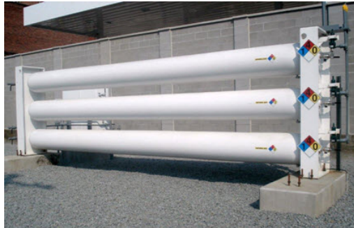
Figure 2(e). CNG Storage Tank
