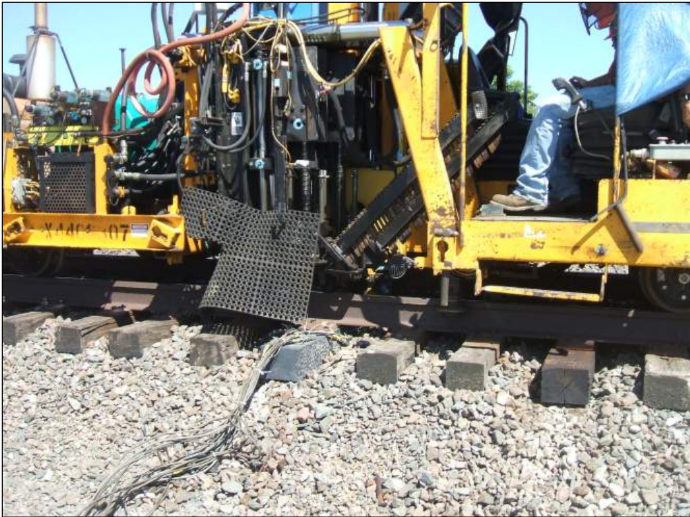
Figure 21. Nipping and spiking operation. The top photo shows the end of the tie bent upwards prior to nipping; the bottom photo shows the tie being straightened out by the nipping and spiking operation.
