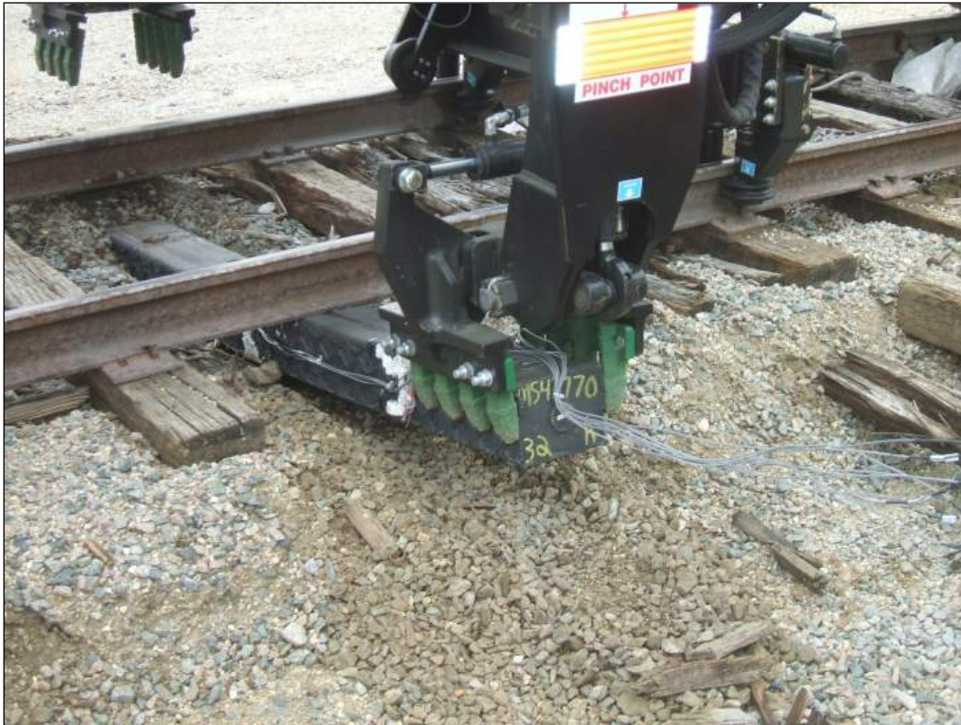
Figure 14. Tie insertion. The tie is bent while digging into the ballast at the far end and being pulled upward against the near rail.
