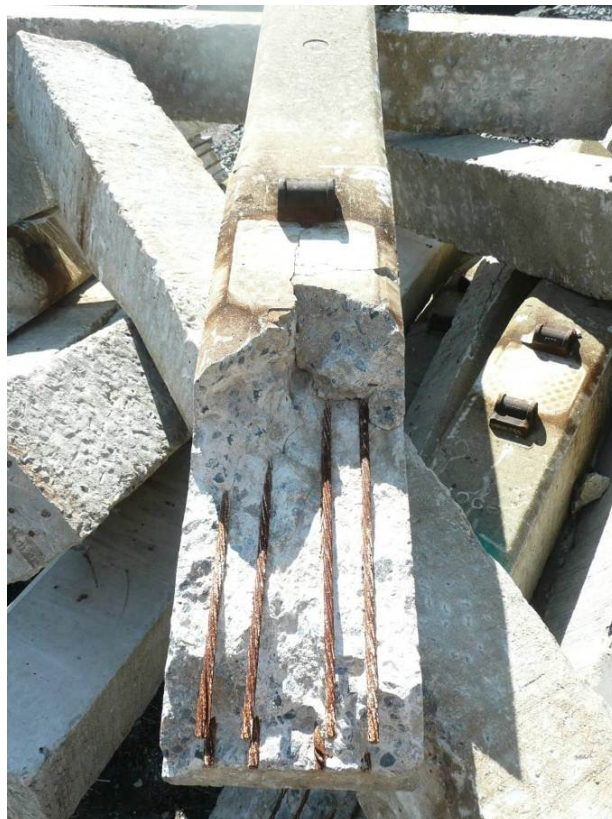
Figure 3.4. An example of a severely cracked tie from the MBTA Old Colony Line.
