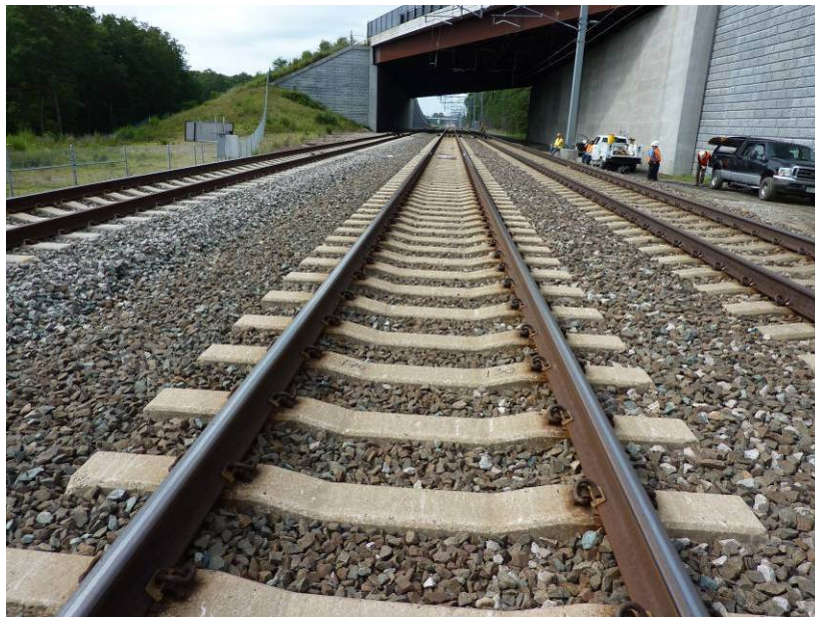
Figure 3.3. A bridge structure near the field test site at which we nondestructively examined ties.
