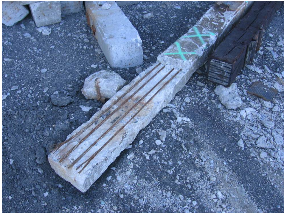
Figure 8.1. A severe example of a tie with the predominant mode of cracking investigated in this study.
