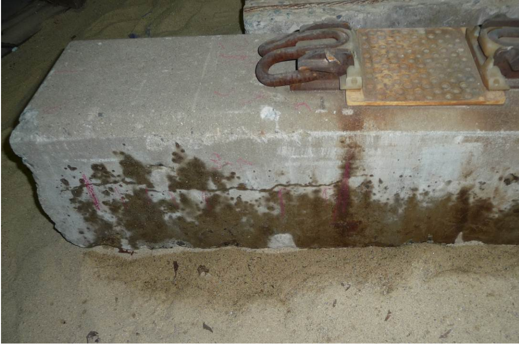
Figure 3.7. Photograph of one of the case study ties showing how the crack is revealed with the use of isopropyl alcohol.
