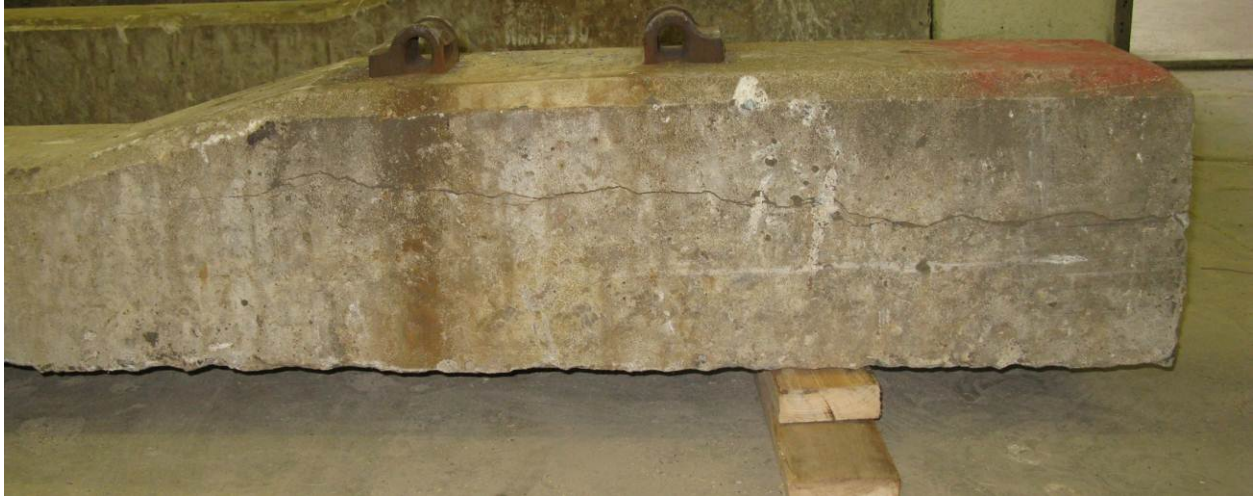
Figure 3.5. An example of a tie with a typical crack from the MBTA Old Colony Line.
