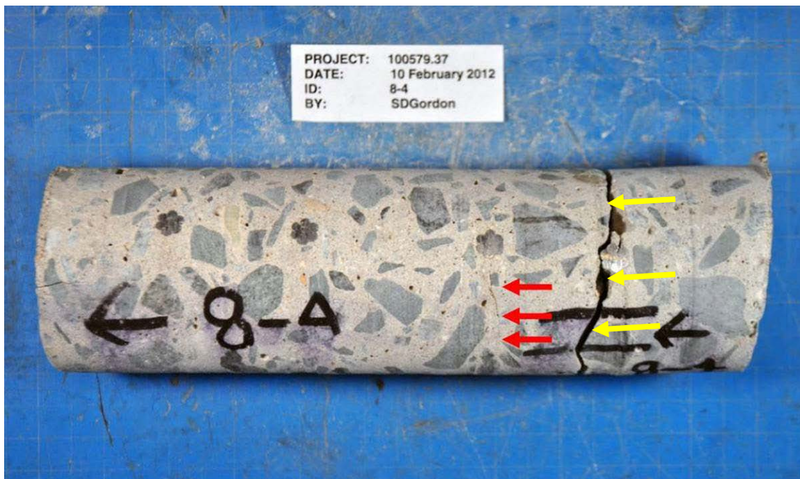
Figure 4.12. Core C8-4 showing the cracks on the circumference of the core sample at tendons (red and yellow arrows). Note: That core fractured at one of the tendons during coring at one of the cracks, thus exaggerating its width (yellow arrows).
