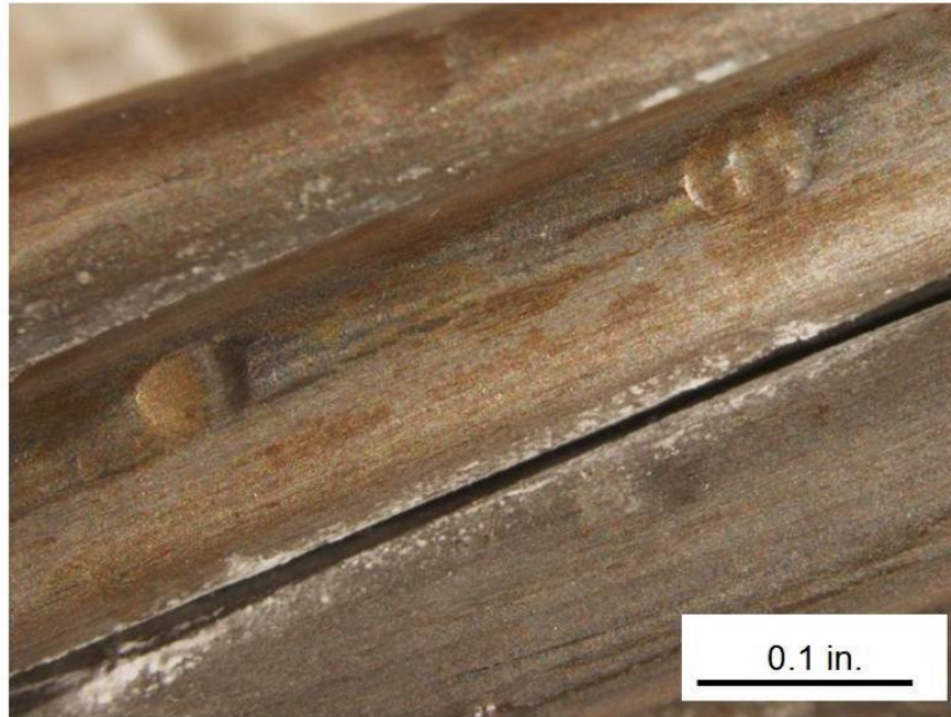
Figure 4.3. Example of elliptical deformations on seven-wire strands from a San-Vel tie.
