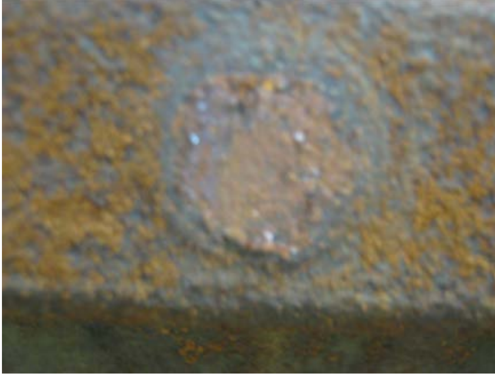
Figure 45. Low Quality IFW Joint due to Misalignment
