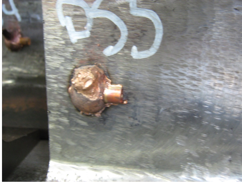
Figure 50. CAD Weld Typical Failure Showing Wire Strand Pullout
