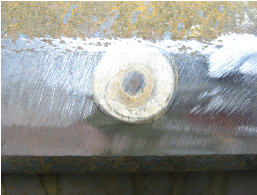
Figure 75. IFW Joint Displaying Evidence of Irregular Surface Preparation
