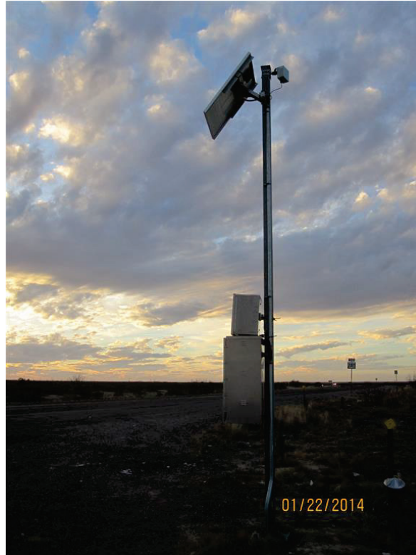
Figure 27. Flasher Cabinet Installed on the Solar Panel Pole.
