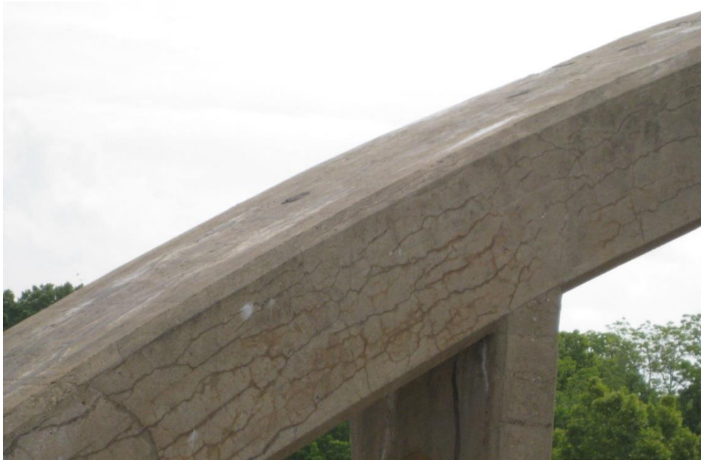
Figure 4: Arch Rib with ASR-Induced Longitudinal Cracks
