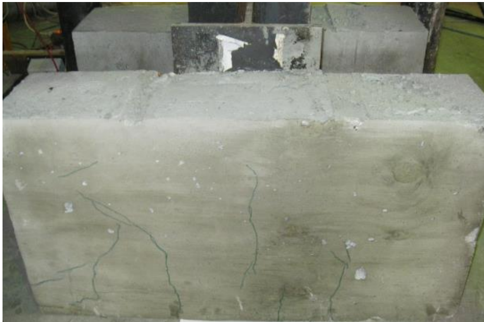
Figure 46. Typical concrete failure (Dang 2013)
