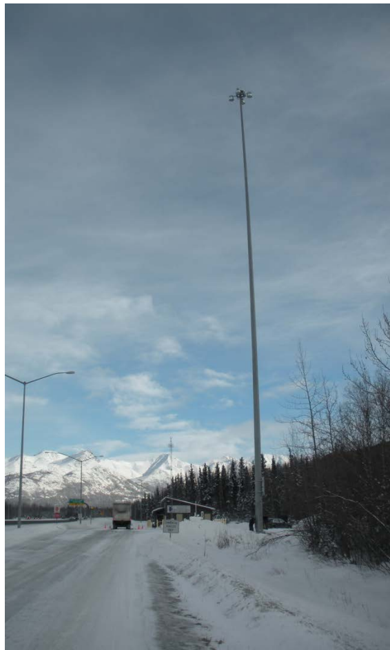
Figure 1.1: A High-mast Light Pole on the Glenn Highway in Alaska
