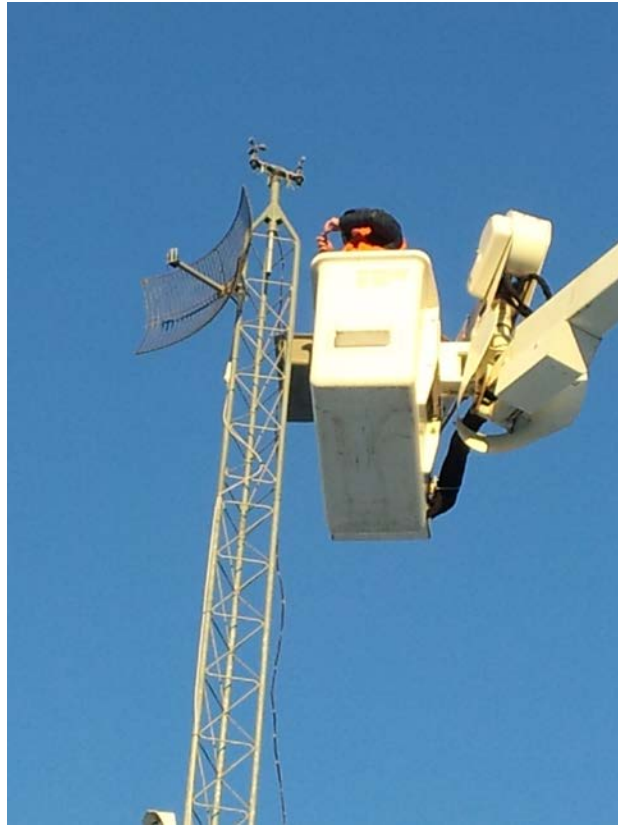
Figure 4.8: Anemometer Installation on Radio Tower at Weighstation
