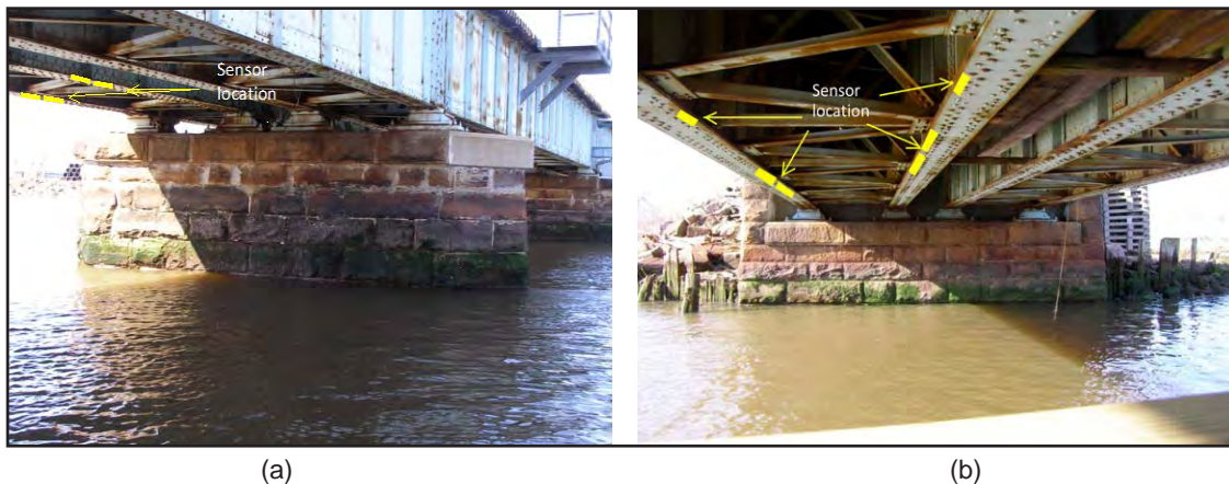
Figure 18. Typical Approach Span (length = 88 ft) of the North Jersey Coast Line MP 0.39 (River Draw) Bridge
