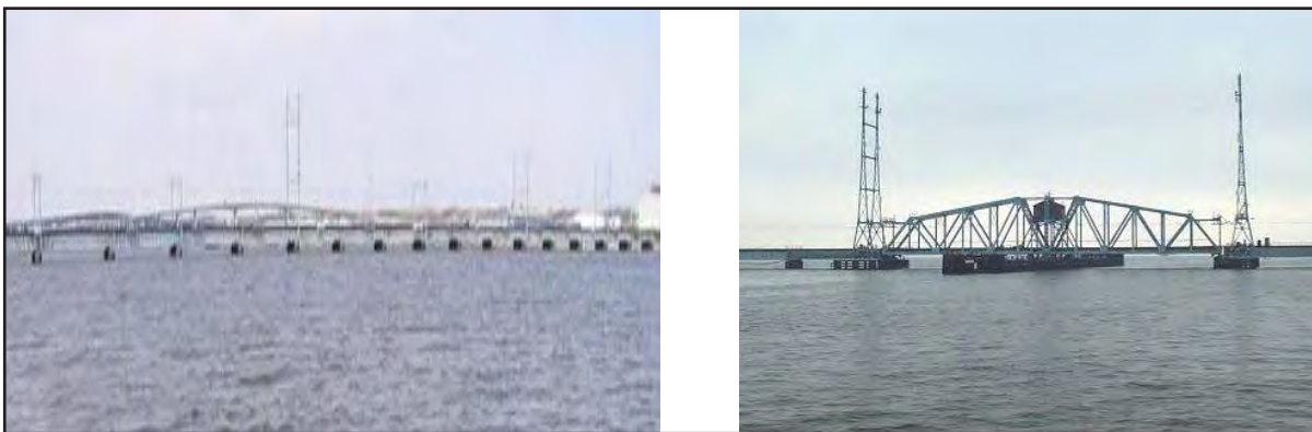
Figure 17. North Elevation of East Approach Span 1 to 18 of the River Draw Bridge
