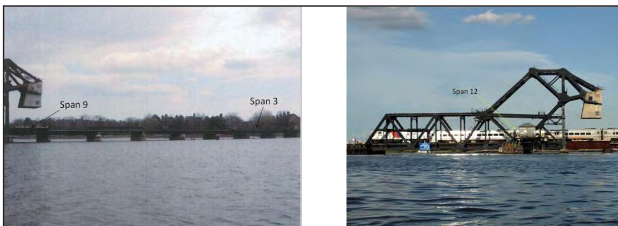
Figure 11. General View of Span 3, Span 9 and Span 12 of the Bergen County Line MP 5.48 (HX Draw) Bridge over Hackensack River Bridge from Inspection Report Cycle 4
