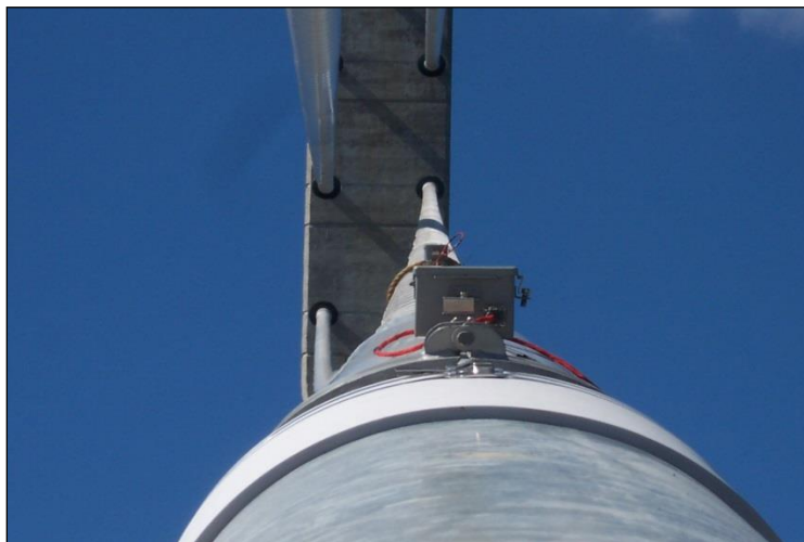
Figure 17. Photo. Accelerometers mounted on stay cable.
