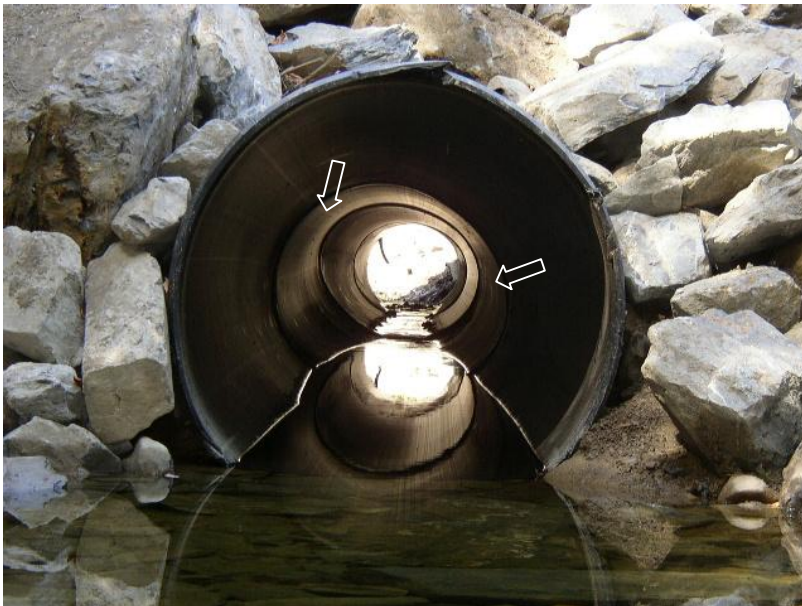
Figure 5 Upstream view of Main Pipe in Benedicta. Pipe is deformed from weight of gravel backfill.
