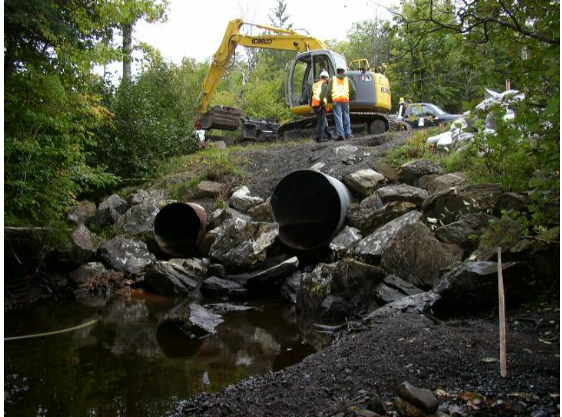
Figure 2 Pre-construction view of cross pipe at Benedicta. New pipe will be installed one foot lower.
