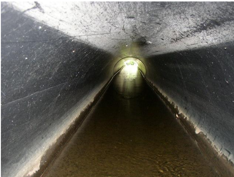
Figure 1 Downstream view of Snap-Tite pipe at Oakfield one year after construction. Center elevation is 4 inches below inlet and outlet.
