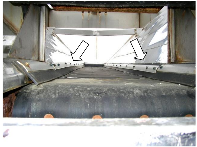
Rubber Strips Used for Confining Salt.
