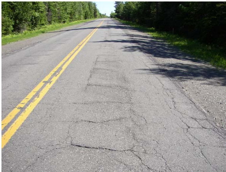
Photo 1: Typical Cracking in the North Lane
