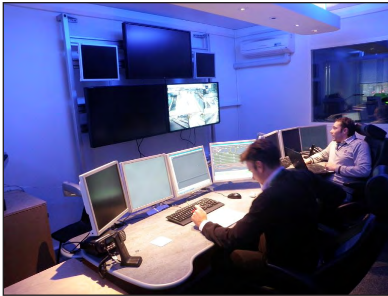
Figure 31. ATN Control Room at London Heathrow Airport
